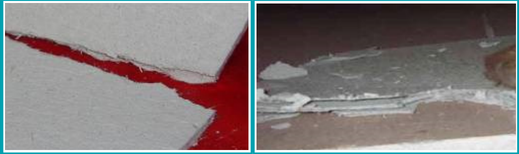
Figure 4 Ragged or torn edges of broken LDB
