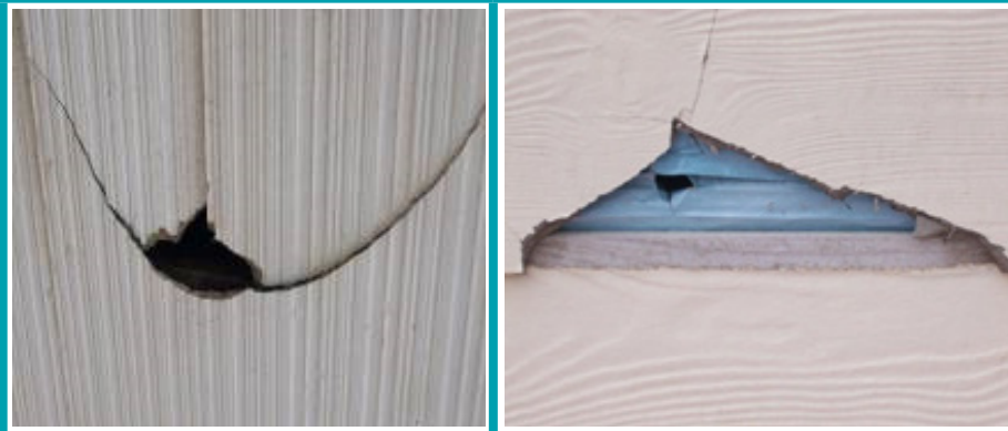
Figure 5 Examples of sharply broken edges on asbestos cement sheeting
