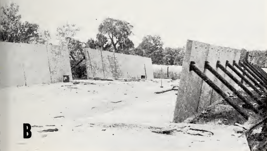
Fig. 7. (A)—Preparing forms for pouring concrete wall panels. (B)—Concrete wall panels in place.
