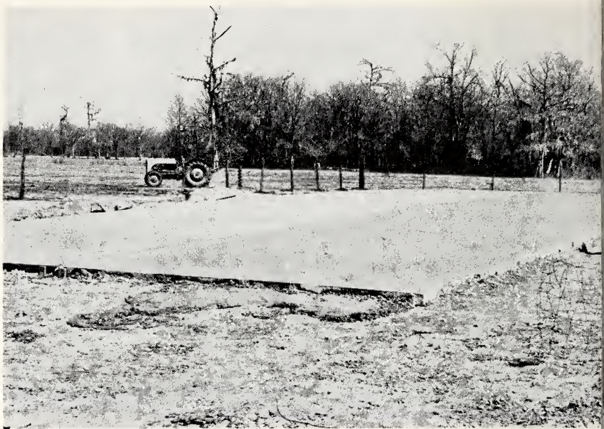
Fig. 1.—Floor slab poured for a bunker silo on a slight ridge in normal flat land.
