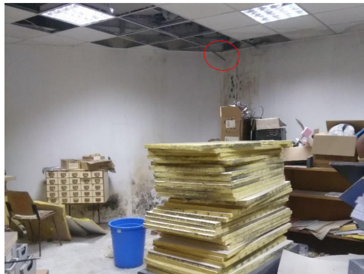
Figure 4.8. The selected area for risk assessment in the Building-C [red circle shows the sampling location]
