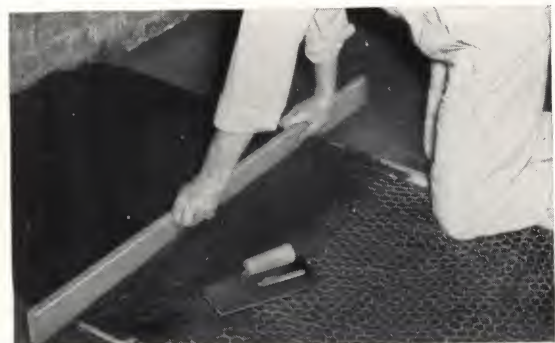
Another method of resurfacing damaged wood and concrete subfloors is the use of a cold mastic floor fill. It can be laid directly over the old floor. Wood screeds and a straightedge may be used to maintain the thickness necessary for leveling. Cold mastic fills will not adhere to subfloors treated with oil. See illustration page 39, top left.
