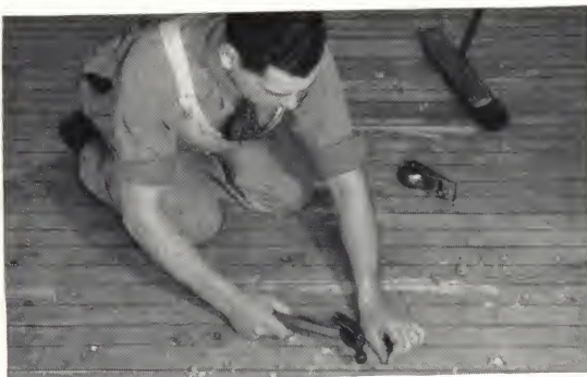
Surface defects in old double wood floors often damage or mar the finished resilient floor. This can be prevented by carefully nailing loose boards and sanding or planing warped areas to floor level. All badly damaged floor boards should be replaced. Sanded areas should be treated with No. S-140 Floor Size.
