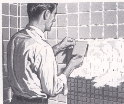
2. Tiles are pressed into the grooves of the foundation board, forcing the grout-adhesive to squeeze out between the tiles into the spaces formed by the tile joints.
