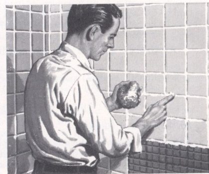
3. Excess grout adhesive is removed and the joints are pointed with a finger. The tiles are then cleaned with a sponge dampened with water or mineral spirits.
