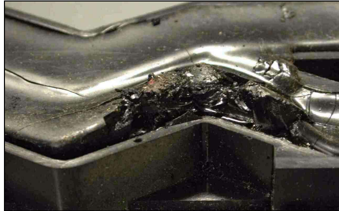
FIGURE 6 - OVERHEATING AT THE CONTACT BETWEEN THE BUSSBAR AND THE STAB SOCKET ASSEMBLY CAUSED THIS DAMAGE TO THE INSULATION. (This view is of the backside of the panel. The damage cannot be seen unless the panel is taken out of the enclosure.)
