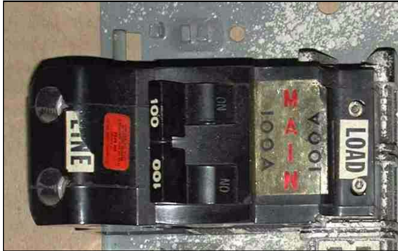
FIGURE 9 - THIS TYPE OF FPE 100-AMP MAIN BREAKER CONNECTS TO THE BUSBARS THROUGH THE PLATE & POST CONFIGURATION, USING ONE SOCKET-HEAD 8-32 SCREW FOR EACH POLE TO ATTACH TO ITS CONTACT PLATE. (The heads of the 8-32 clamping screws are seen at right, above and below the "LOAD" label.)
