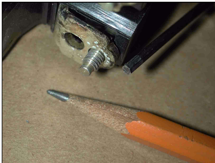
FIGURE 10 - ONE LOAD-SIDE CONTACT AND ITS 8-32 CLAMPING SCREW, ON THE FPE 100-AMP MAIN BREAKER OF FIG. 9. THE SCREW-HEAD TAKES A 3/32" ALLEN WRENCH, WHICH IS ONLY SLIGHTLY LARGER THAN THE LEAD OF THE PENCIL. (The larger hole next to the clamping screw provides clearance for the end of the screw that protrudes from the mating contact plate)
