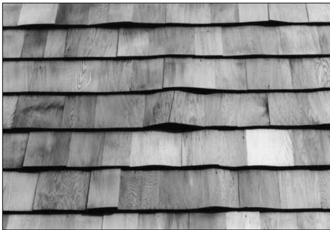
Figure 7. Buckling of shingles installed with insufficient gap.
