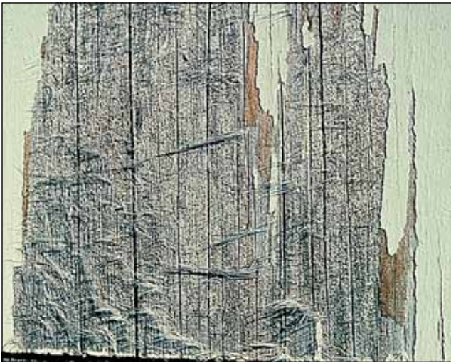
Figure 17. Severely weathered wood surface.
