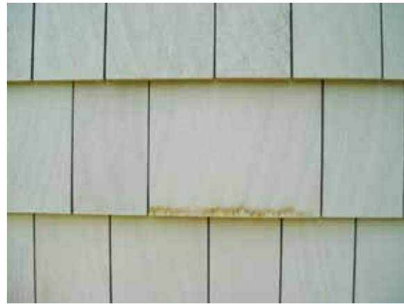
Figure 15. Single coat of solid-color stain. Note the extractives bleed.
