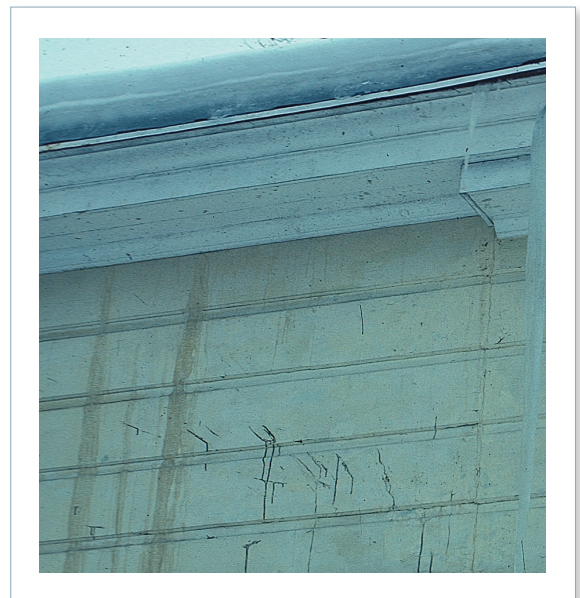
Figure 4 —Ice dam on roof and gutter. The resulting water intrusion into the wall and behind the siding often causes run-down extractive bleed.
