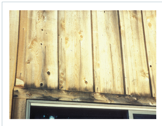
Figure 3 —Extractive bleed from end-grain absorption of water. Note the fasteners have also caused iron staining.
