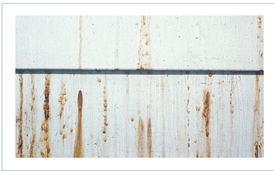
Figure 2 —Run-down extractive bleed.
