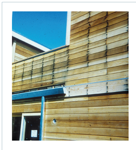
Figure 8 —Iron stain on newly constructed home. The intent of the owner was to have a natural finish (lightly pigmented semitransparent stain) on the siding. To correct this, the siding will need to be replaced.
