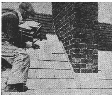
Figure 14. Proper flashing at all intersections is important.
