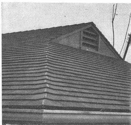
Figure 39. Simple "laced" hip and louvered gable. Louvers should be screened and provided with movable doors.
