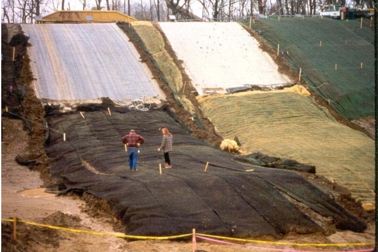
Figure 3-23. Photograph of slides in plot G (left) and H (right) taken approximately 2 months after construction and several days after the slide in plot G.
