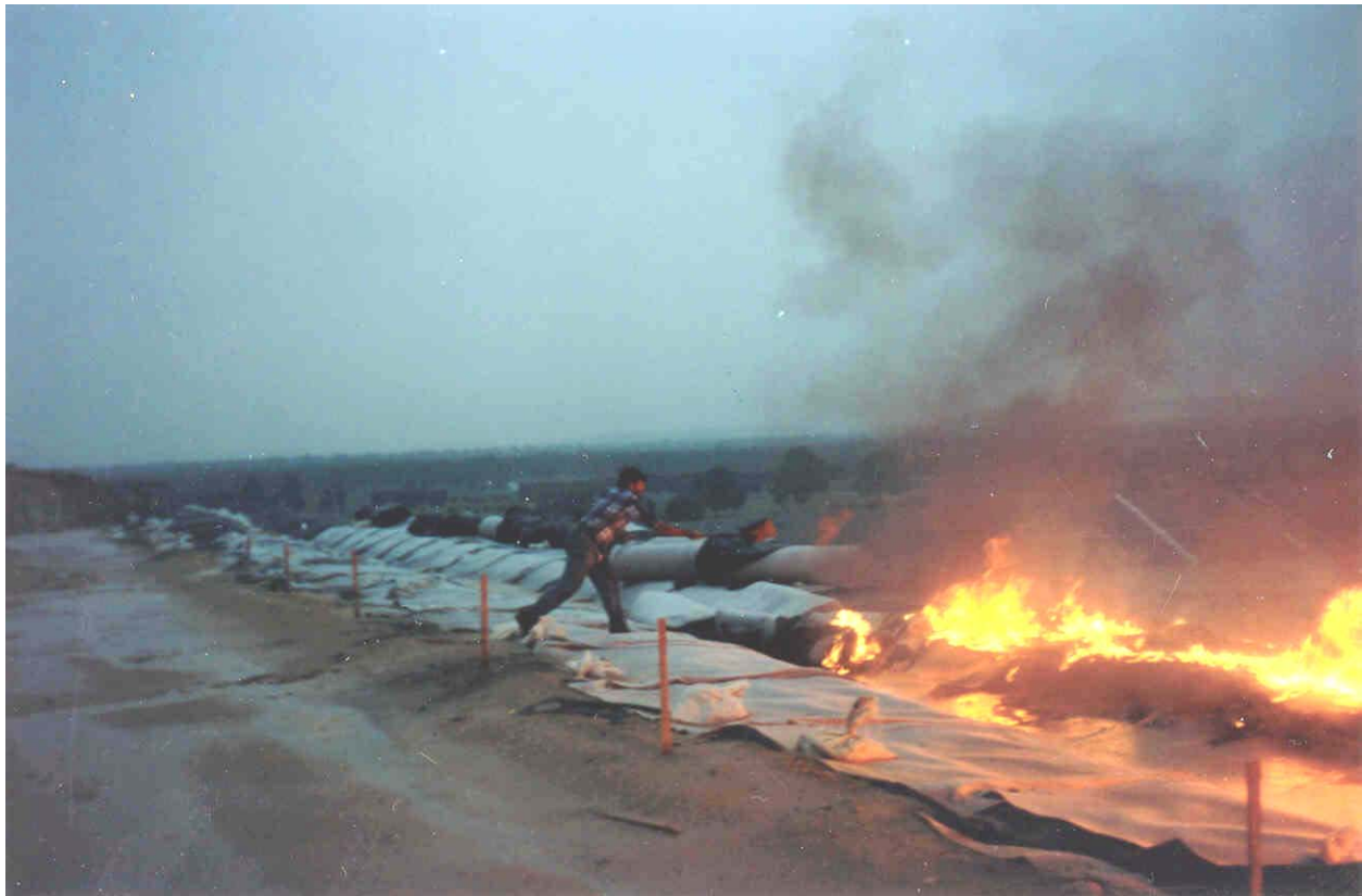
Figure F-A.3.1. GC rolls at the top of a liner system side slope caught fire (potentially due to a lightning strike) and damaged the underlying GM.
