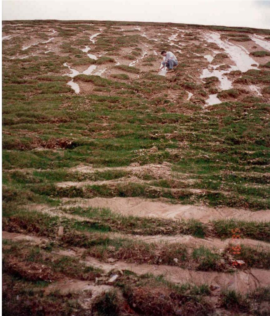
Figure F-A.12.1. Cover system at the end of the second sliding episode.
