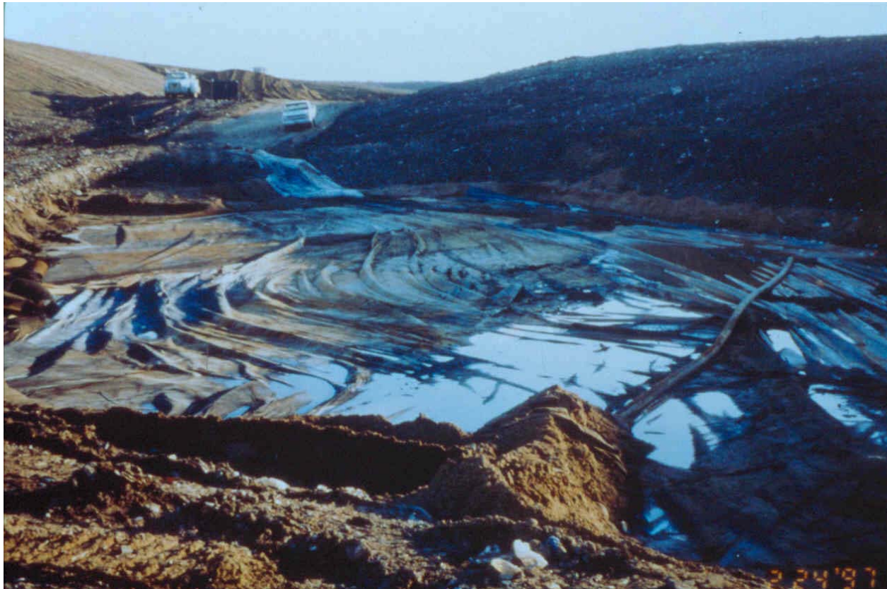
Figure F-A.8.1. When waste was excavated from the failure zone, large wrinkles in the GCL were evident.
