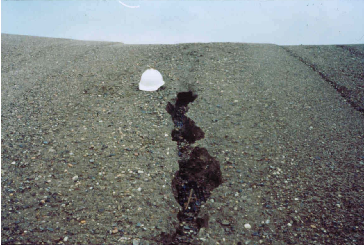
Figure F-A.2.1. Construction debris in a CCL with an initially smooth surface protruded from the CCL after the CCL was left exposed and subsequently eroded.
