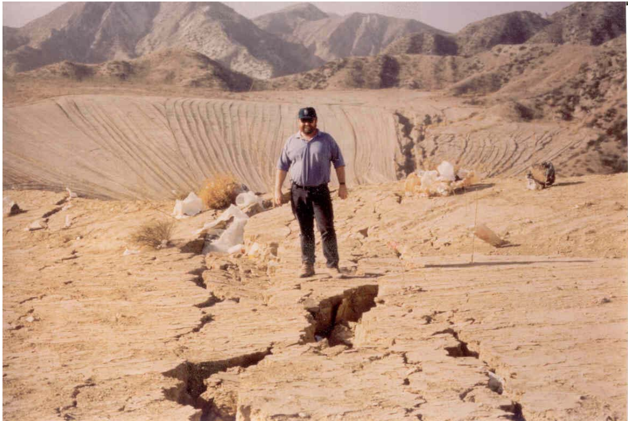
Figure F-A.8.2. Longitudinal cracks in soil intermediate cover at Chiquita Canyon Landfill after the Northridge earthquake.
