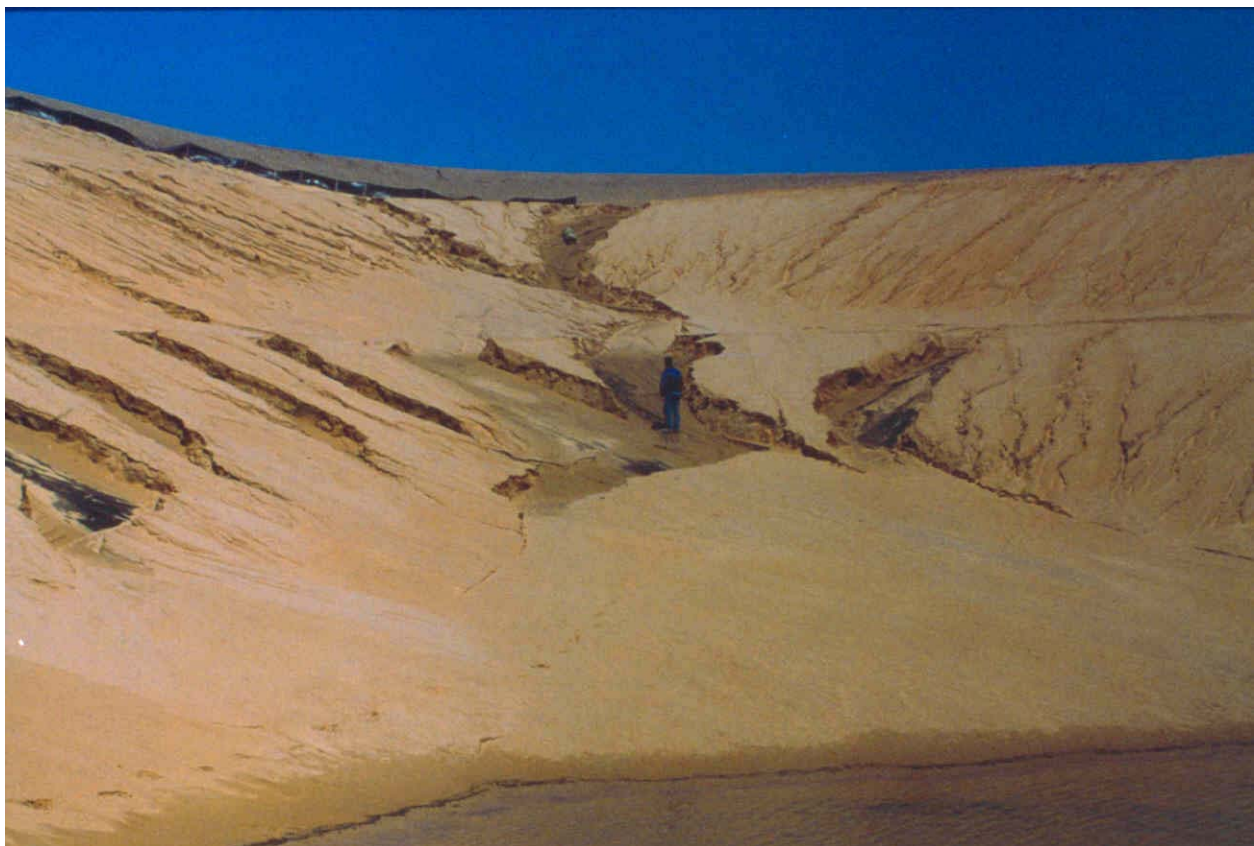
Figure F-A.5.1. Erosion of sand protection layer on liner system sideslopes.
