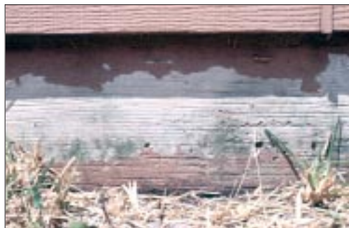
Masonite says faulty installation and maintenance caused problems with its product in South Florida. The siding shown here was installed in contact with the ground.
