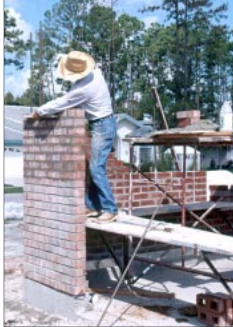
SuprKing structural bricks are slightly oversize and have large holes for grout and rebar. Here a mason works on a reinforced load-bearing brick wall.
