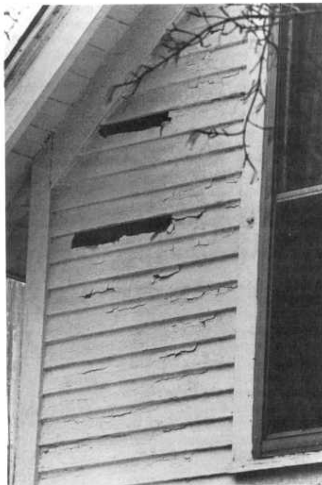
Figure 35 —Paint peeling from wood can result when excessive moisture moves through the house wall. Some cross-grain cracking is also evident on this older house.
