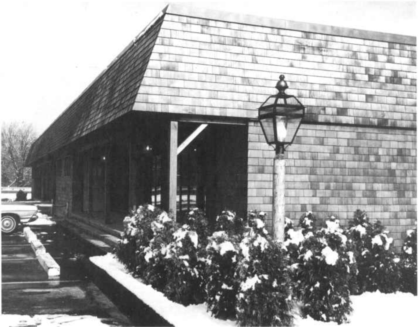
Figure 27 —Application of wood shingles to a commercial structure. (Photo courtesy of the Red Cedar Shingle and Handsplit Shake Bureau)
