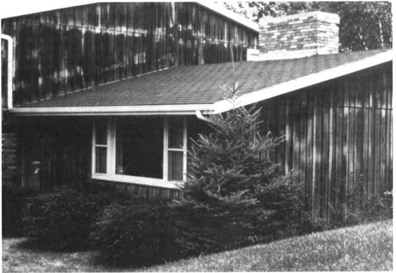
Figure 26 —Lap marks formed by improper application of a semitransparent penetrating stain.
