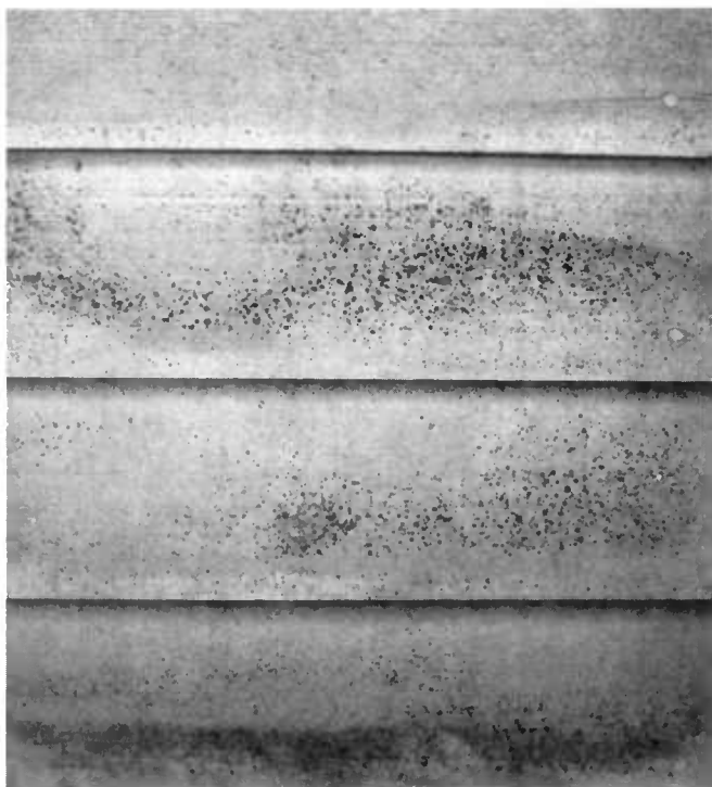
Figure 31 —Mildew on paint is most common in warm humid climates as well as in shaded or protected areas.
