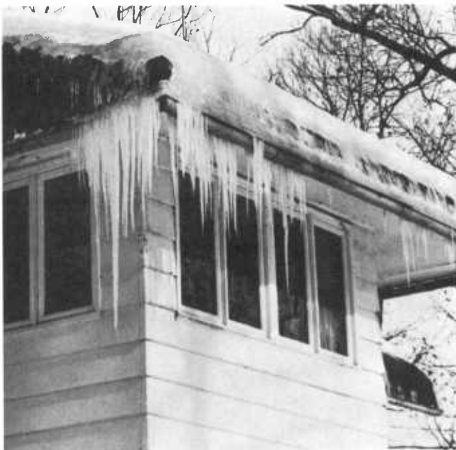
Figure 5 —Ice dams in cold climates causing severe moisture problems in roofs, ceilings, and walls. Peeling paint and extractive staining may result.
