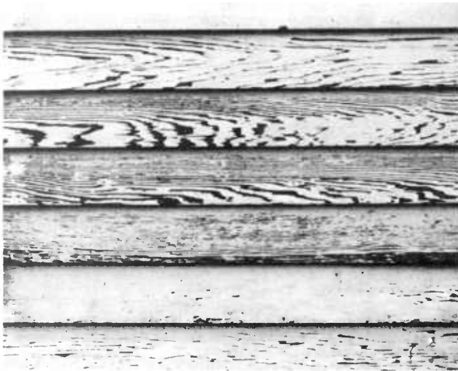
Figure 12 —Paint applied over edge-grained boards (top and bottom). It performs better than that applied to flat-grained boards (middle).
