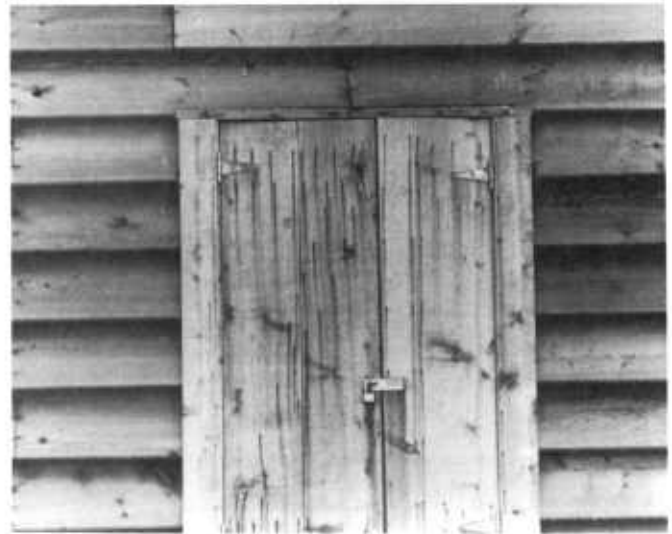
Figure 39 —Blue-black discoloration resulting from the use of ferrous nails.
