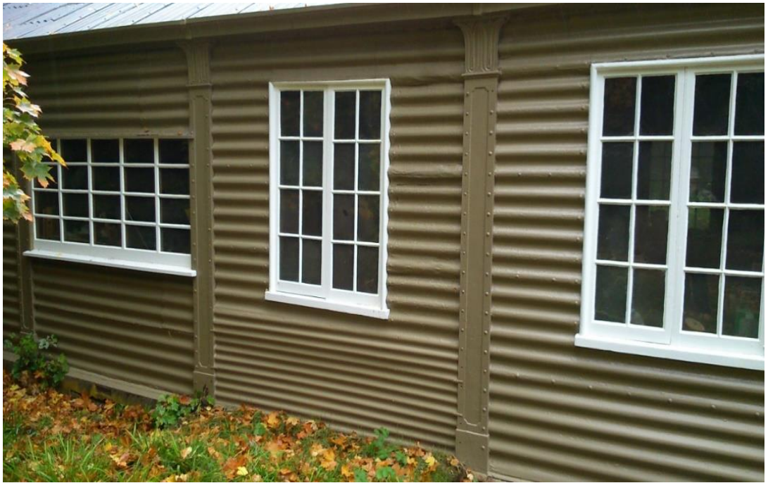
Figure 4.17. Recent repairs to the ballroom using steel. Modern, steel-based, corrugated iron has been used to repair the lower part of the central panel. This repair is probably connected to the removal of the original door and its replacement by window. It is not clear how the narrow pitch of the repair corrugated iron has been matched to the profile integral to the cast iron frame.
