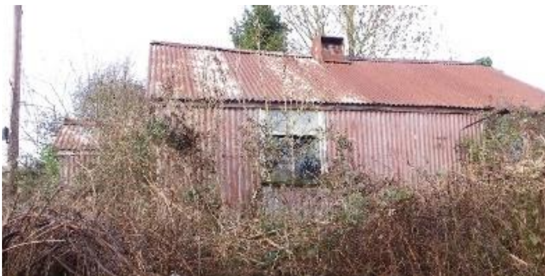
Figure 3.14. An abandoned corrugated iron chapel at Rodhuish in Somerset. Its designation and at-risk status is unknown, but if it remains unoccupied and unmaintained its life expectancy is very limited in this condition. Photograph by the author.
