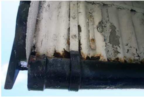
Figure 4.30. The condition of the corrugated iron in the underside of the eaves illustrates the generally poor condition of all the roofing sheets. The only area where repair rather than replacement was deemed impractical was the roof, where there was extensive damage to the corrugated iron. Severe corrosion had taken place at the lower edge where the corrugated iron came into direct contact with the cast iron guttering and its fixings; also damaged by corrosion was the joint between the ridge piece and the roofing sheets. Photograph by Sonya Linskaill.
