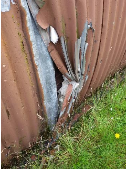
Figure 4.52. Every aspect of the site provides difficult maintenance challenges. This damage has been caused by an accidental impact from a ride on lawnmower. Such incidents are probably inevitable when the Comrie Development Trust Has to rely on volunteer labour for grounds maintenance. The damage reveals that the underlying corrugated iron is in surprisingly good condition, but unless repairs are carried out swiftly water ingress will do rapid damage. Photograph by the author.
