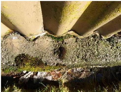
Figure 4.58. One major problem, found on many of the huts, is the reinforcement of the lower edges of the corrugated iron with bricks and concrete. This has been poorly executed and is trapping water between the concrete and the metal which will accelerate corrosion of the corrugated iron. Photograph by the author.
