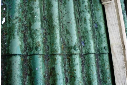
Figure 4.29. Corrosion protection: This image shows the failure of more recent paint on the roof. Although the underlying paint film appears to be largely intact, and there is no evidence that the galvanising has failed, this still needs attention. Most importantly, it looks horrible and is an invitation for any hostile fewer to suggest that the whole building needs demolition. Technically this failed paint is trapping water which is likely to speed up corrosion of the underlying metal. Photograph by Sonya Linskaill.
