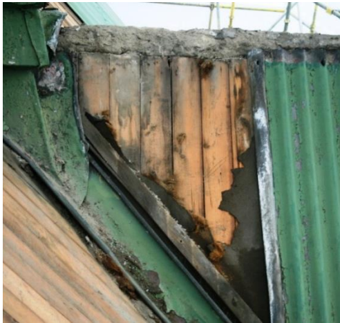
Figure 4.42. Glass fibre insulation introduced into the airspace between the corrugated iron and the internal timber boarding when the eastward extension was added in the 1960s. Such insulation carries a severe risk of timber decay and cladding corrosion because it restricts the ventilation. Omitting new insulation emphasises that the repairs have sought to preserve the authenticity of the building, and by doing so to maintain its cultural significance. Photograph by Sonya Linskaill.
