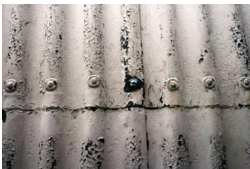
Figure 4.37. A peculiarity of St Fillan's is the quantity of fixings used to secure the edge of walling sheets. It is highly unusual to nail in the trough of every corrugation as has been done here. This oddity would seem to match the poor quality of the roof board meeting (see above) and is another indication of an inexperienced being used to erect the church. Photograph by Sonya Linskaill.
