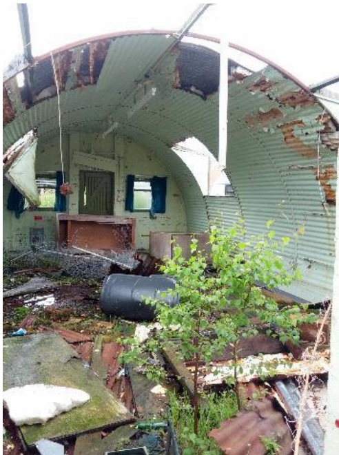
Figure 4.51. The climate at Cultybraggan is particularly hostile, with high rainfall, extreme cold, and strong winds. Wind, especially, will have damaged the huts by driving moisture between the lap joints of each corrugated sheet. The internal corrosion visible here had started before the corrugated iron cladding and lining had been cannibalised to repair other huts. Photograph by the author.
