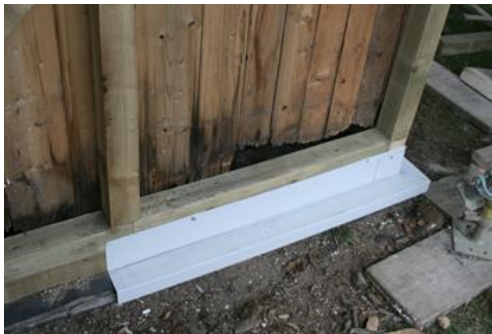
Figure 4.36. A particular vulnerability of prefabricated corrugated iron buildings is rainwater removal from the lower edge of the walls. Conservation at St Fillan's has departed from the original design and improve the drainage detail by inserting a preformed metal sill behind and under the corrugated iron. Photograph by Sonya Linskaill.
