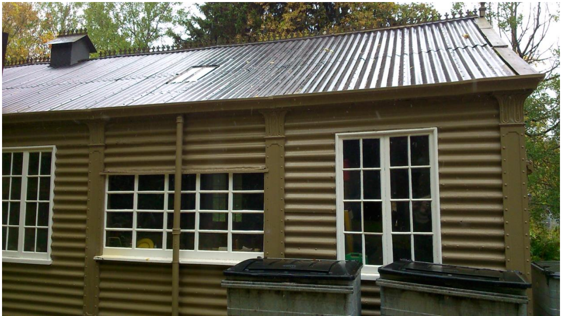
Figure 4.15. Window detail of the ballroom. The windows are all softwood replacements, except for two longer and lower windows (one shown centrally in this image) the form of the replacements appears to follow the original design. The paint condition is variable and needs maintenance.
