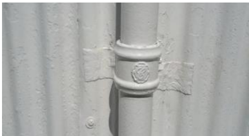
Figure 4.39. Patch repairs to localised corrosion damage caused by the electrolytic reaction between the cast-iron of the downpipe and the galvanised steel corrugated cladding. The repairs been formed in glass fibre and there is a risk of ultraviolet light attack. Care will be needed to keep them well painted in order to prevent this. Photograph by Sonya Linskaill.
