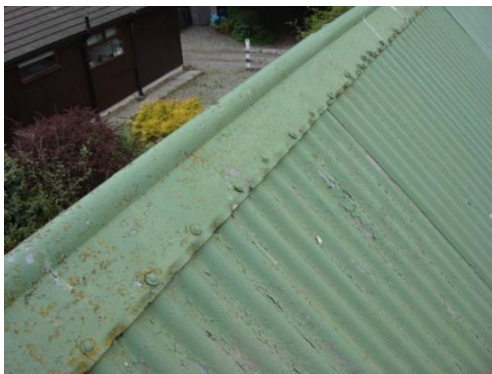
Figure 4.31. Ridge piece (at top of roofing sheets). Dismantling showed that significant amounts of water had entered the roof because of the poor quality of this detail. There is a poorly shaped lap between the ridge piece and the roofing sheets. Photograph by Sonya Linskaill.
