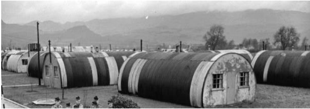
Figure 4.61. Repairs to the corrugated iron. The paler sections are where new sheets have been introduced to repair corrosion damage, and not as was suggested by Heritage Group volunteers, markings to prevent attack by Allied aircraft. The date of the repairs is not known, but probably the 1960s. Image from Comrie Development Trust.
