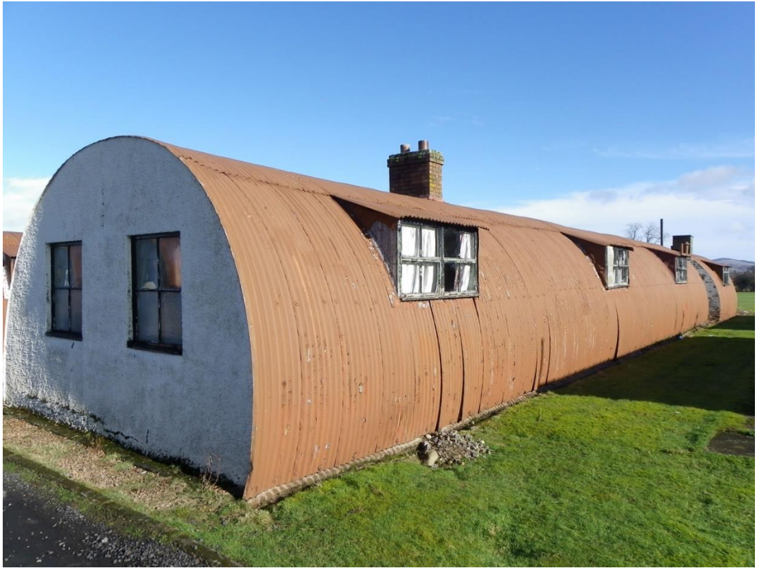
Figure 4.49. Corrugated iron Nissen hut at Cultybraggan. The Camp preserves an extraordinary example of corrugated iron architecture's survival; but this survival does not mean that it can be easily conserved. Although huts like this appear to be in reasonable condition, hidden defects in the framing, heating system combine with the need for external maintenance to make conservation a daunting task. Photograph by the author.
