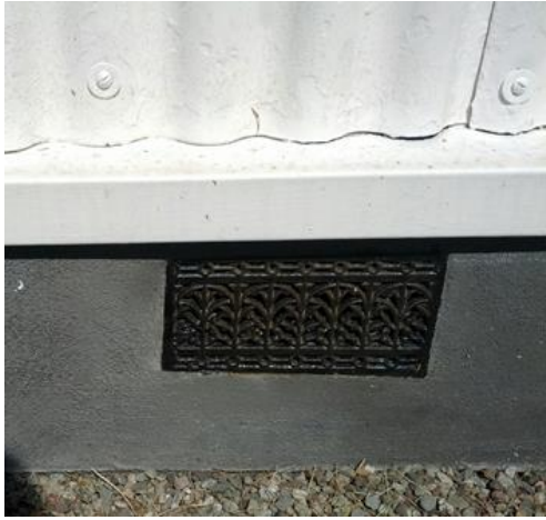
Figure 4.41. A metal cover has been added at the bottom of the wall-sheets to throw condensation and rainwater clear of the brick plinth. The rainwater down-pipes have been modified to connect closely with newly installed drains. Just as importantly the original cast-iron ventilation grills have been cleaned and repaired to continue subfloor ventilation to the interior. Photograph by Sonya Linskaill.
