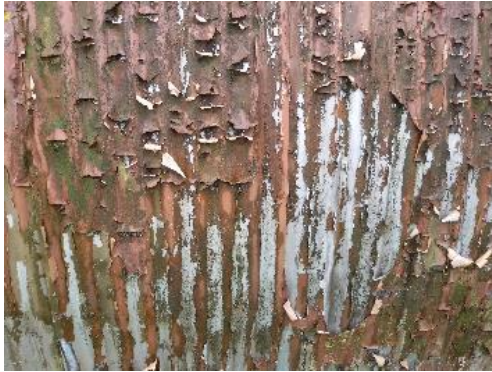
Figure 4.55. The three-year gap between the end of military use and the takeover by the Comrie Development Trust, was a damaging break in repainting and general maintenance and has caused major paint failures. These failures are starting to permit corrosion of the corrugated iron. Photograph by the author.
