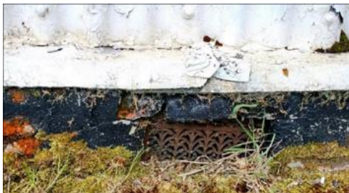
Figure 4.35. Detail of the lower edge of the wall cladding, showing how condensation and leakage has decayed the lower rail of the structural framing and allowed the wall to sag. Photograph by Sonya Linskaill.
