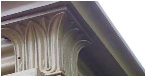
Figure 4.13. Frame detail of the ballroom. The frame has no significant decay problems and has good paint adhesion.
