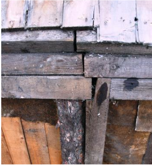
Figure 4.34. This image illustrates the prefabricated framing of St Fillan's. Each prefabricated section of the walls had a square frame butted against its neighbour. The image is complicated by the paler section of wood (middle left, under the upper wall plate) which appears to be a replacement.
