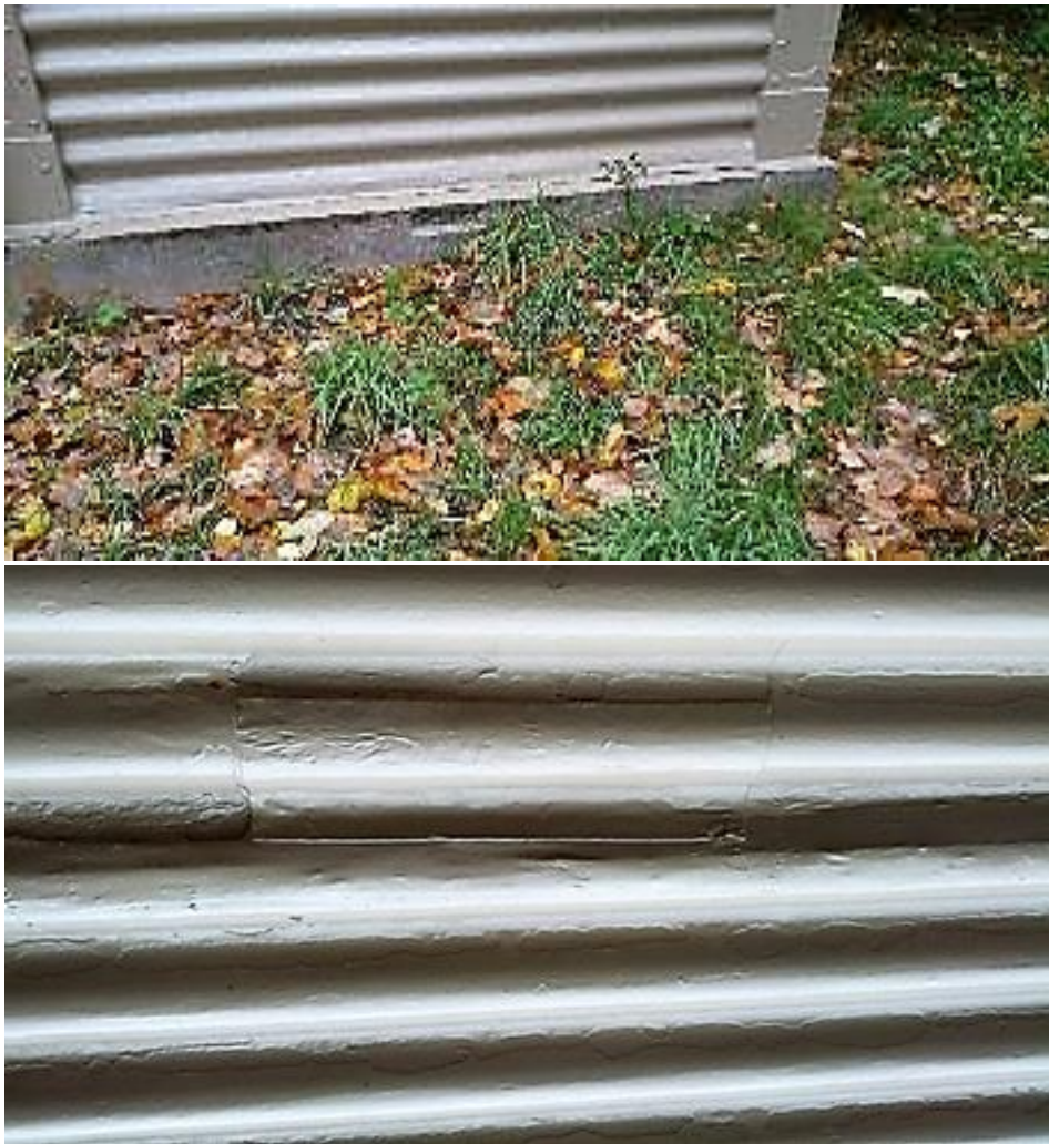
Figures 4.18 and 4.19. Repairs to corrosion damage using glass fibre reinforced resin. Though skilfully done, the change in surface texture caused by these repairs is noticeable. Against these disadvantages resin repair is cheap and highly weather resistant in the short and medium term. It is relatively easy to remove and retreat and allows the maximum retention of historic material. Balancing the pros and cons of conservation strategies is rarely straightforward.
