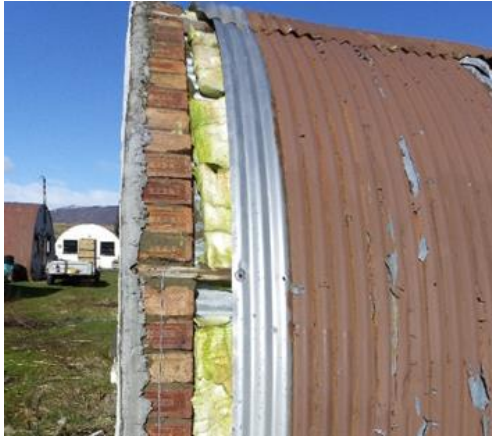
Figure 4.63. Military attempt (probably from the 1980s) to introduce insulation between the corrugated iron skins. Note the excellent condition of the corrugated iron exposed by removal of the closing sheet. This is clearly a modern replacement that calls into question the authenticity of much of the site.
