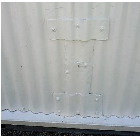
Figure 4.40. Patch repairs are nailed to the original corrugated iron. These appear to have been done at some considerable time in the past. It is not clear how well they have been waterproofed all-weather matching corrugated iron for the patches was obtained. They do, however, appear to be working satisfactorily. The conservation approach to the repair at St Fillan's has not chosen to make good pre-existing repairs, but to retain them. Photograph by Sonya Linskaill.
