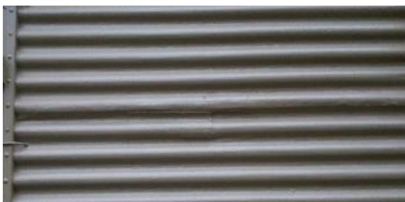
Figure 4.14. Original wrought iron corrugated panels on the walls. In generally excellent condition with only light surface corrosion pitting. This suggests that paint film maintenance has not always been consistent.
