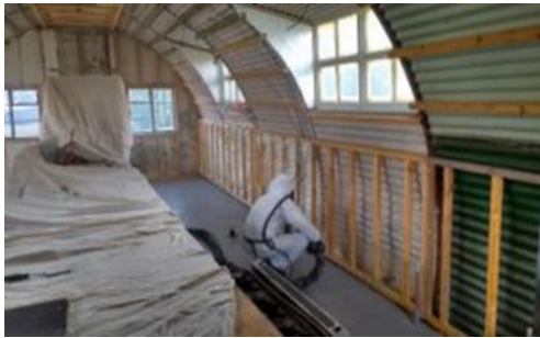
Figure 4.64. The refurbishment of two Nissen huts that will be used as part of the museum, housing the Heritage group's collection and the visitor's centre. The original corrugated iron lining has been retained and it will be interesting to see if condensation problems interfere with the museum displays. Image from Comrie Development Trust.
