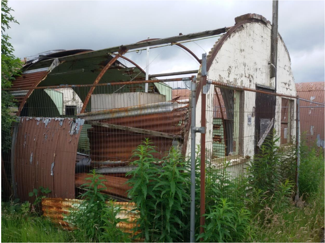
Figure 4.50. The poor condition of many of the huts, partly due to the quality of the materials used. The steel and the galvanising are likely to have been compromised because of wartime shortages, and because the buildings were only seen as temporary. Photograph by the author.
