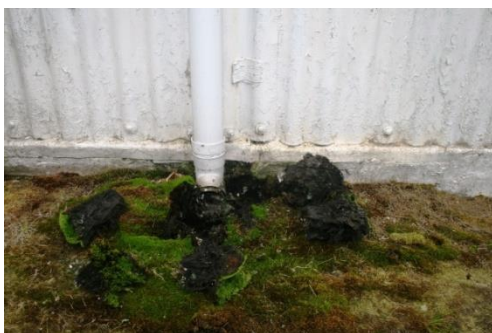
Figure 4.32. Before repair, the downpipes appeared to be working correctly but discharging directly into the soil adjacent to the walls. This was causing excessive moisture to be drawn into the plinth wall, the civil beam of the wooden frame and the lower edge of the corrugated iron, causing them all to decay. Conservation often fails to see beyond the immediate object, but in this case the architect has installed a functioning subsurface drainage system. The drain is now repaired and functioning correctly. An interesting conflict arose between the architect and building control over the proposed installation of a French drain. Such drainage systems are a commonplace in conservation specifications but were not acceptable to the local building control officer. Photograph by Sonya Linskaill.
