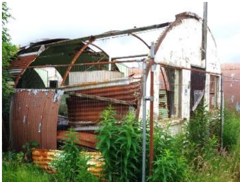
Figure 4.56. Cannibalisation has revealed the frame of this hut emphasising that the corrugated iron is more or less self-supporting, and the main function of the frame is to tie the sheets together rather than holding them up. The render here has failed primarily because thermal expansion of the corrugated iron relative to the masonry has stressed it to breaking point. Photograph by the author.
