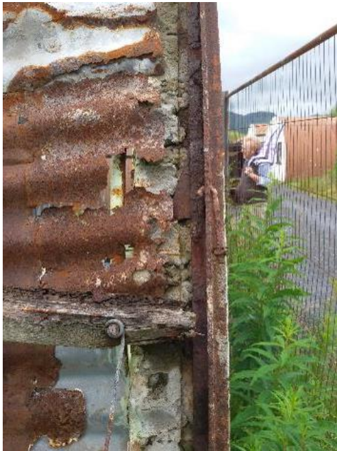
Figure 4.53. A further vulnerability of the basic design is the termination of the corrugated iron at the end walls. This has yet to be satisfactorily addressed. Water penetrating along and through the end wall is trapped between the masonry and the corrugated iron causing rapid decay of the metal. Photograph by the author.
