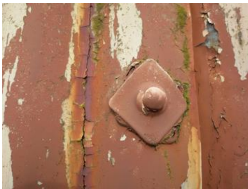
Figure 4.54. Though not the case here, fixings generally are a source of water ingress. Thermal expansion of the corrugated iron is a real problem, and fixings have to be flexible enough to accommodate this without coming loose. This is a major challenge and the fixings frequently fail in the long term. Photograph by the author.
