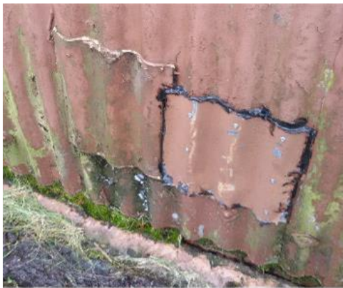
Figure 4.60. Patch repairs are attractive from a conservation point of view because they involve the minimum loss of original material. Here, however, they depend on the cannibalising of other huts to obtain the patch material and the use of potentially corrosive metal fittings to secure the patch. Adding a sealant to make the patch waterproof is essential, but there is no reason to do it as unattractively as this. Photograph by the author.
