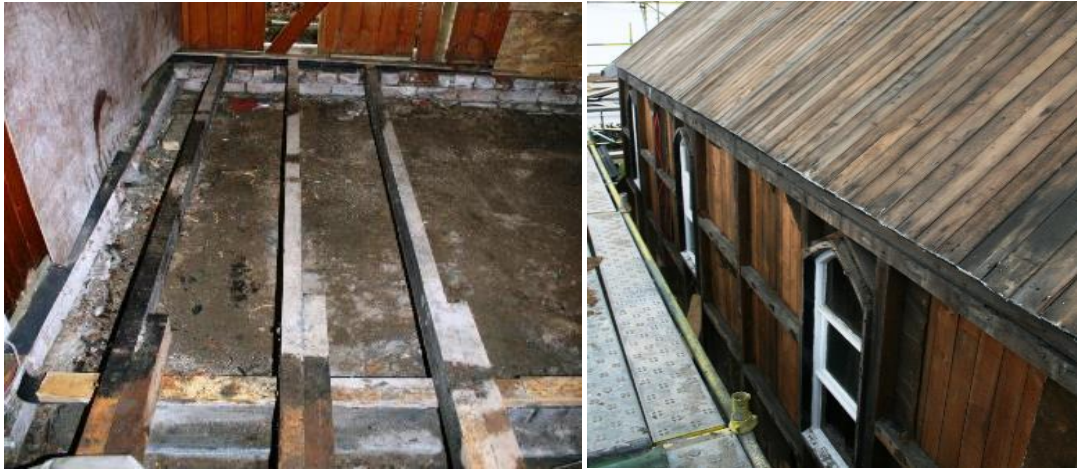
Figure 4.33. Details of wooden frame. St Fillan's follows the standard nineteenth century approach to constructing corrugated iron chapels. This used a wooden frame to support (and be stiffened by) the corrugated iron cladding. In this way an air gap is automatically created between the corrugated sheets and the internal timber boarding. The gap allows ventilation which minimises the build-up of condensation on the inside face of the corrugated iron and thus produces a durable form of construction. Historically, this durability depended largely on the high quality of timber used in the framing. The durability of the wood masked a fundamental problem: corrugated iron sheeting is inherently prone to accumulate condensation on its inner surface. The quality of wood currently available to repair the original framing does not match that of the original. Photographs by Sonya Linskaill.
