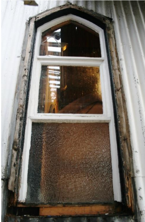
Figure 4.38. One of the nave windows during dismantling of the church. Note that the glazing is applied to a fully finished subsidiary frame and not directly to the wall framing that surrounds it.
