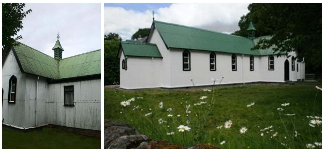
Figure 4.28. A general view of the church before and after repair. Note the dark staining at the lower edge of many sheets of corrugated iron. This is caused by biological growth which is benefiting from moisture trapped in the lap of the sheets. It is a sign that the corrugated iron is not seating well and is allowing moisture penetration. The general dowdiness indicates that the paint needs renewal. Photograph by Sonya Linskaill.
