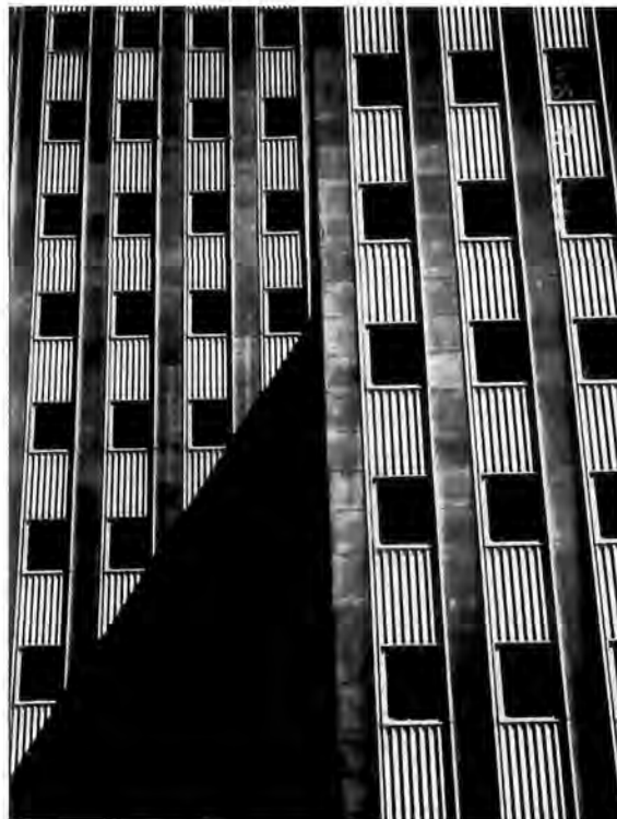
Fig. 3. An early aluminum curtain wall used in conjunction with the then more traditional limestone curtain wall. The fluted aluminum spandrel plates and center pivot windows have contributed to water leakage over the years.
