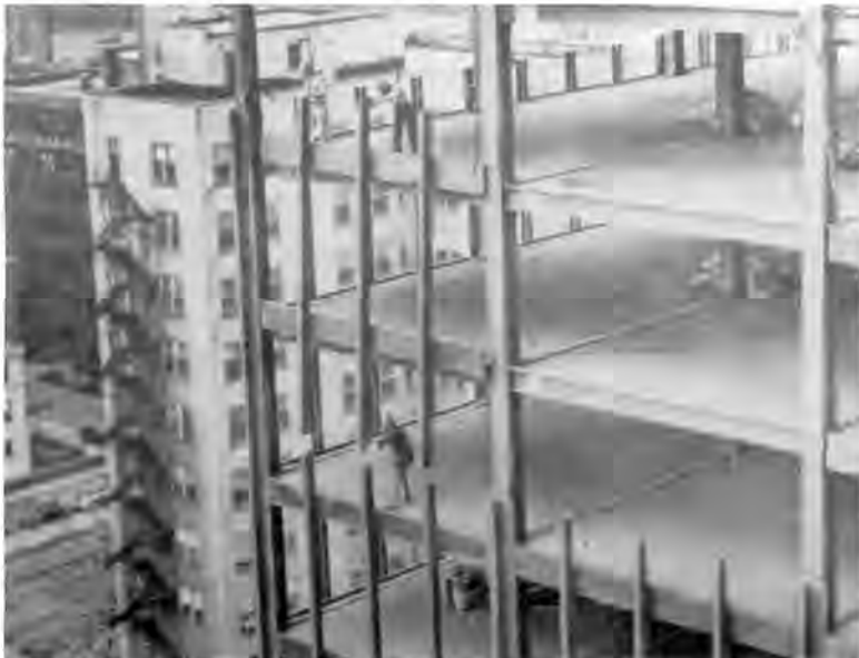
Fig. 1. Construction photograph of 860-880 Lake Shore Drive apartment buildings, Chicago, Illinois (Mies van der Rohe, 1949-1951). These were among the first residential buildings in the United States to be clad entirely in glass, with a two-story prefabricated steel and aluminum curtain wall system.
