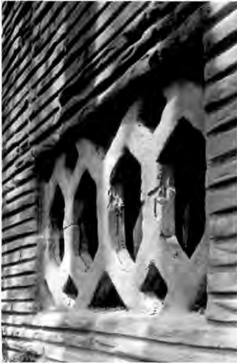
In 1950 the Wieboldt-Rostone House was covered with Perma-Stone, shown in poor condition. Photo by Jack E. Boucher, HABS, NPS.
