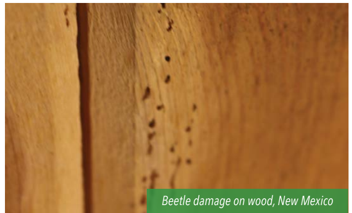
Powderpost beetle carcasses and frass in a crawlspace, New Mexico
