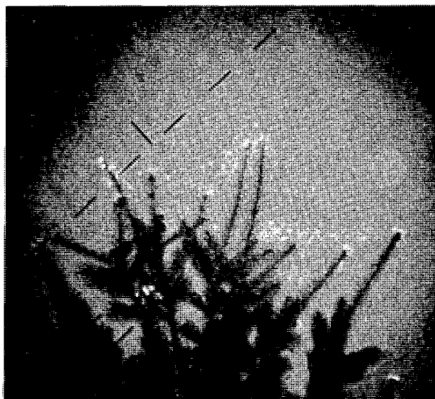
FIGURE 14. Induced corona on a Douglas-fir tree purposely left growing close to the BPA 1200-kV prototype line. The same effect also occurs if trees grow too near 500-kV or 765-kV lines. Photograph taken with a night vision device.
