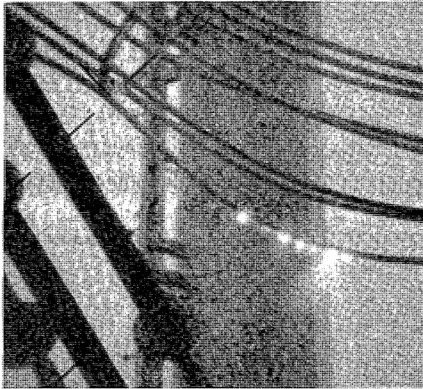
FIGURE 41. Corona visible on conductors of the 1200-kV prototype line. Photograph taken with a night vision device.
