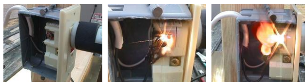
Fig. 8 Ground fault receptacle, with glowing contact, on fire
