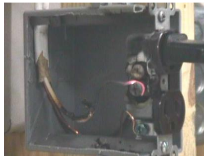
Fig. 6 Glowing contact on duplex receptacle neutral terminal
