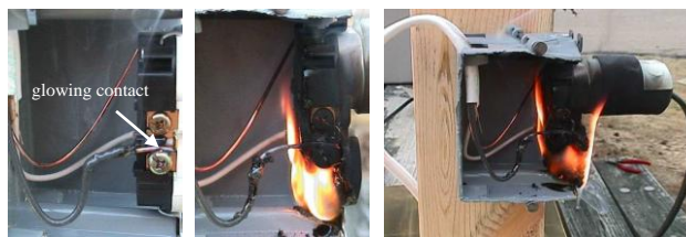
Fig. 7 Duplex receptacle, with glowing contact, on fire
