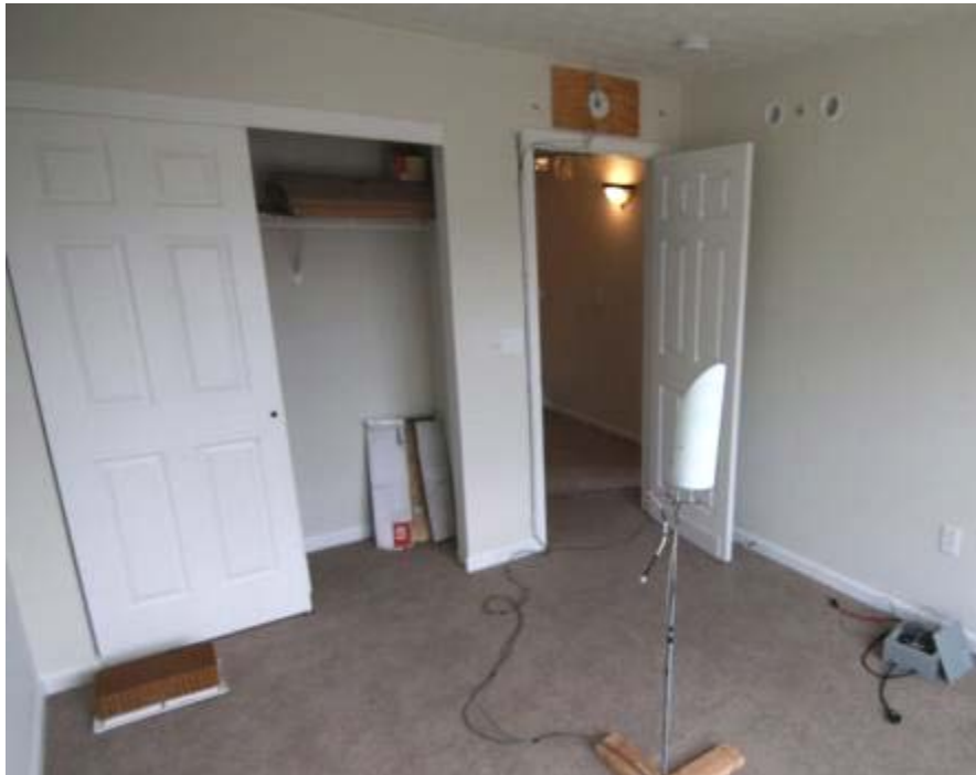
Figure 3. Photograph from the interior of bedroom 3 showing the supply outlet and air temperature measurement stand
