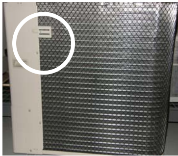
Outdoor air temperature sensor
