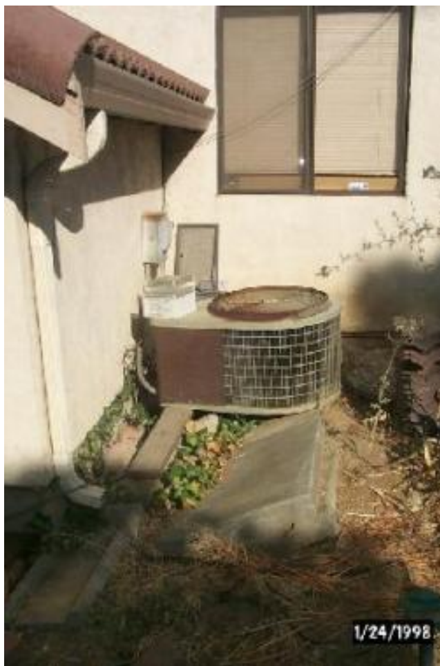
A good candidate for replacement: an old condensing unit showing poor condition of unit (heavily corroded sheet metal and fasteners and significant dirt/dust blocking flow into coil) and subsided slab (that we believe led to stresses on refrigerant lines with a subsequent leakage of refrigerant – this system had too little charge)
