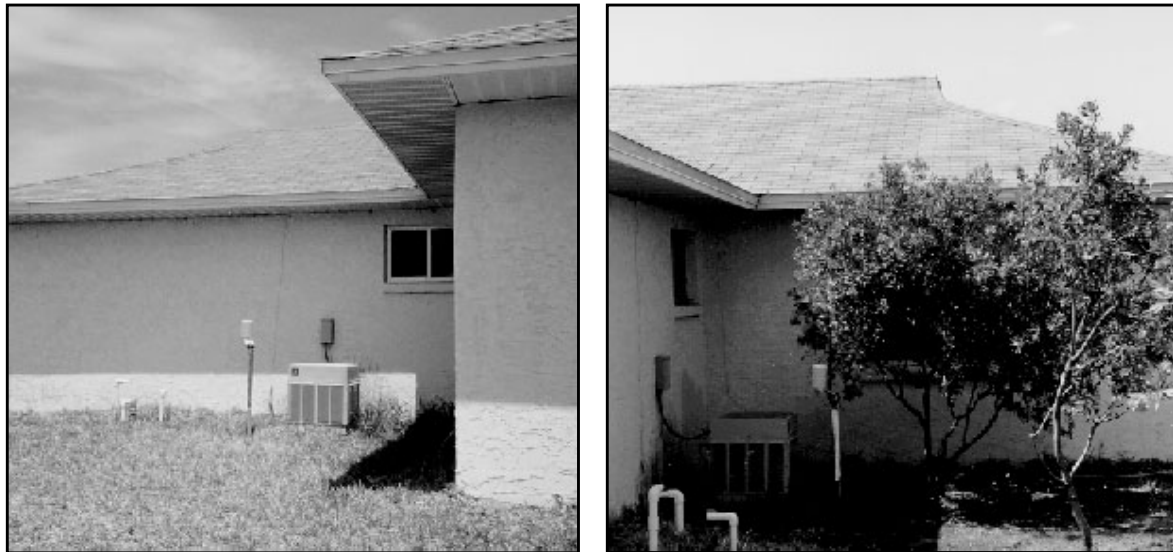
Figure 3. West-Facing Condenser at Site 1 Prior to Landscaping (Left); Final Appearance after Tree Planting (Right)
