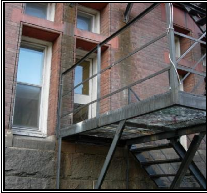
Figure 105: Rust runs down the masonry facade; anchorage many have weakened (author, 2005)
