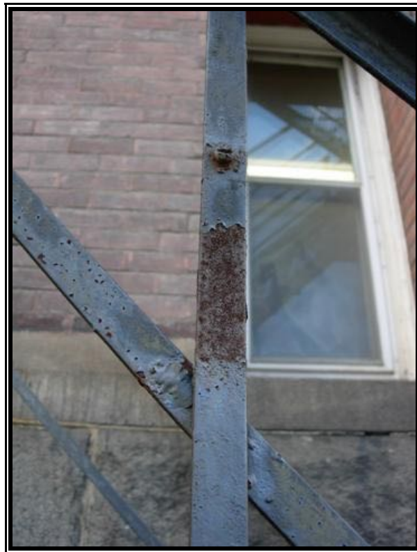
Figure 111: Rust that can be scraped and primed and painted (author, 2005)
