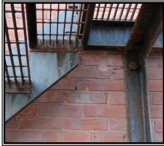
Figure 108: Deteriorating stair treads and bracket (author, 2005)
