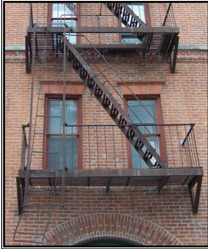
Figure 112: Drop ladder is bent out of shape and unusable (author, 2004)
