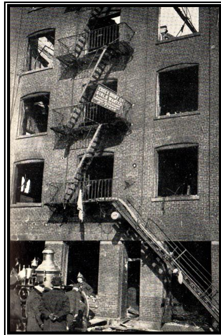
Figure 22: Flames shot out the window at this deadly factory fire, rendering the fire escape impassible. (“Two Factory Fire Holocausts,” Quarterly of the National Fire Protection Association 9 (1916), 273.)
