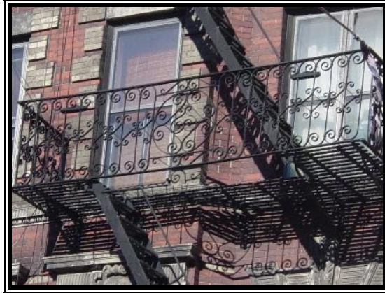
Figure 118: Ornamental fire escape at 169 Sullivan Street, South Village, New York City (Greenwich Village Society for Historic Preservation, “South Village - A Distinguished History Largely Unrecognized,” New York City, http://www.gvshp.org/south_village948.htm )
