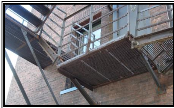
Figure 109: Broken balcony railings (author, 2005)
