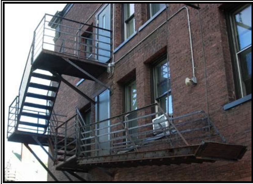
Figure 110: Severely rusted drop ladder; hinge probably stiff (author, 2005)
