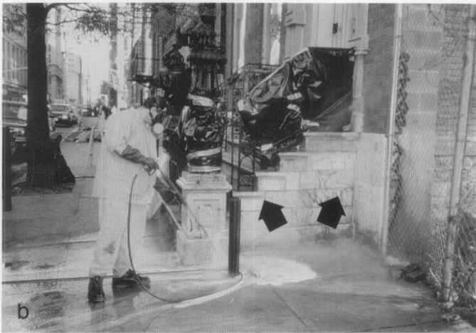
Figure 4 (a-b). After cleaning with an alkaline paint remover, remnants or ghosts of black spray-painted graffiti are still visible and may require poulticing, while the blue paint has been almost completely removed. Photos: Mark A. Weber.
