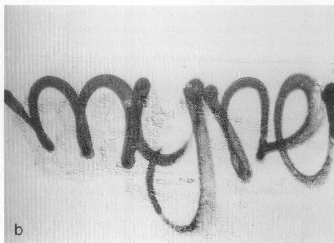
Figure 7 (a-b). The first time this spray-painted graffiti appeared it was removed abrasively. As a result, the graffiti was permanently etched into the limestone and cannot be concealed even by the pigmented barrier coating painted over it later. The barrier coating did, however, facilitate non-abrasive removal of graffiti the next time it was applied. Photos: Anne Grimmer.
