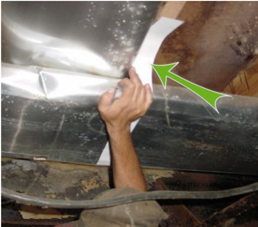
Secure sagging ductwork
