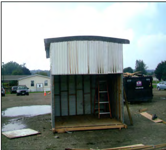
The main reconstruction project, the tool shed; 12 feet high by 6 feet wide.
