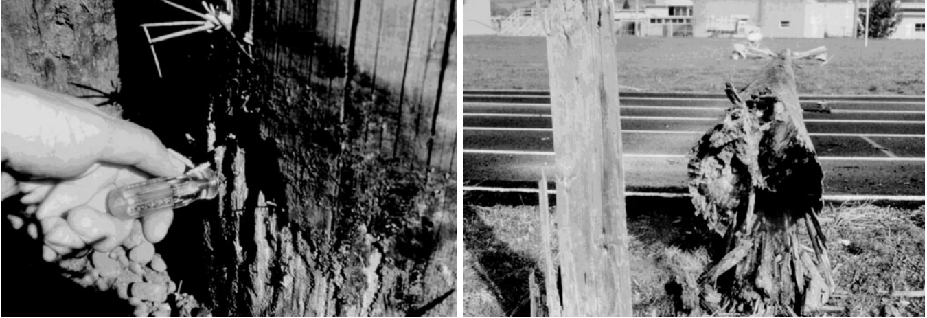
Figure 22. External (left) and internal decay (right).
