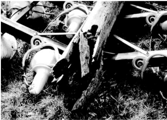
Figure 4. Decay in a field-drilled pole.
