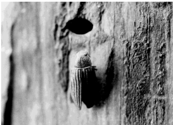
Figure 17. As an indication of internal rot in the above-ground portion of poles, look for the oval holes, 1/2 in. long, that the buprestid beetle leaves as it emerges from wood. Many holes could mean an unsafe pole.
