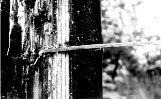
Figure 25. A shell-thickness indicator detects rot in poles by “feeling” growth rings in sound, but not rotten, wood when inserted or removed from snug-fitting holes.
