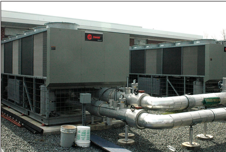
Figure 5-3. Air-Cooled rooftop chiller in Georgetown, Delaware.
