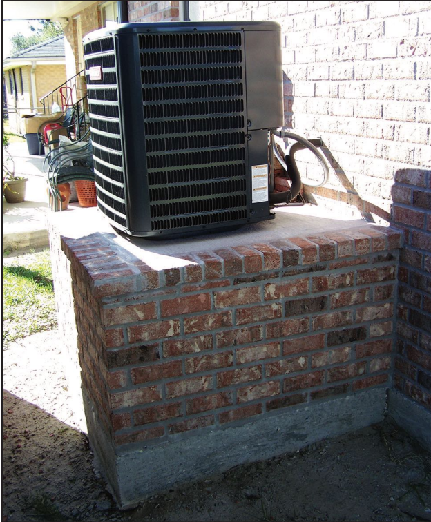
Figure 3-1. Air conditioning compressor elevated on a pedestal.
