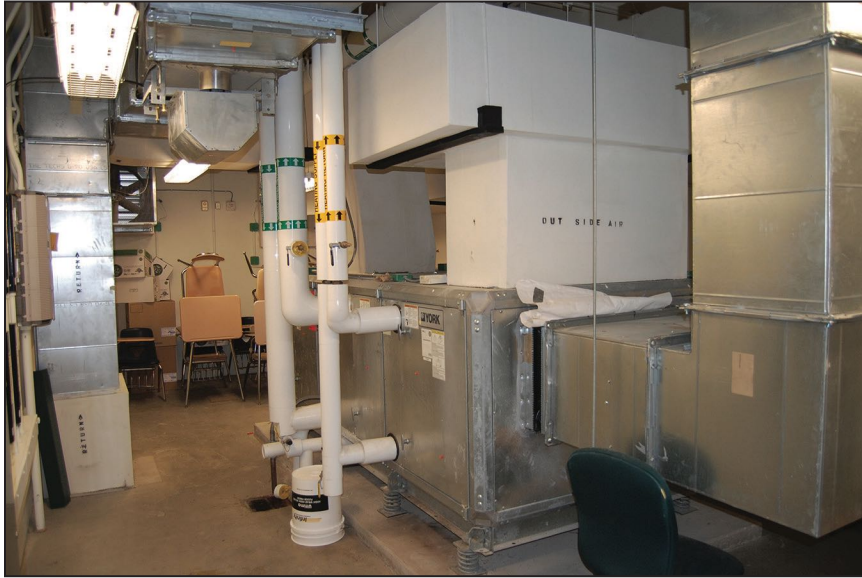
Figure 5-6. AHU with a separate chilled water coil (green labels) and hot water coil (yellow labels). The coils are within the unit and are not visible (Dagsboro, Delaware).
