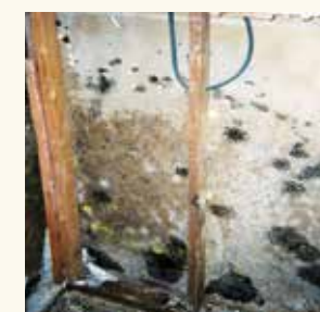
PHOTO 1: Mold and rot from leaving wet insulation in wall.
