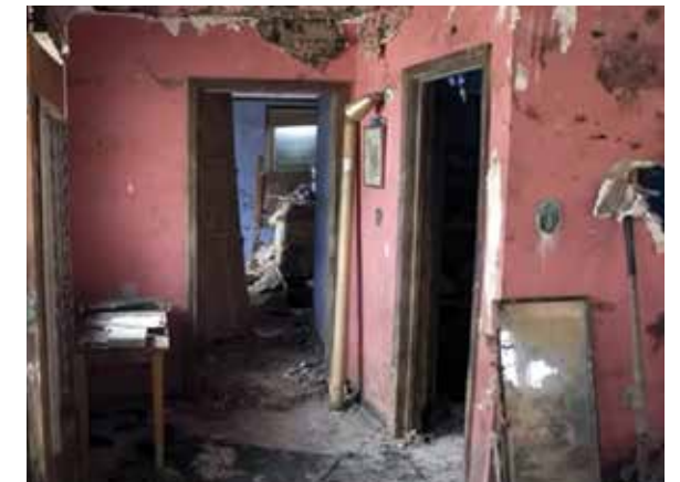
PHOTO: Remain alert to hazardous walking and working conditions.
