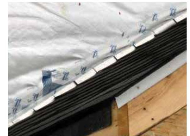
PHOTO: A water-resistant barrier layered over step flashing at a roof-to-wall intersection.
