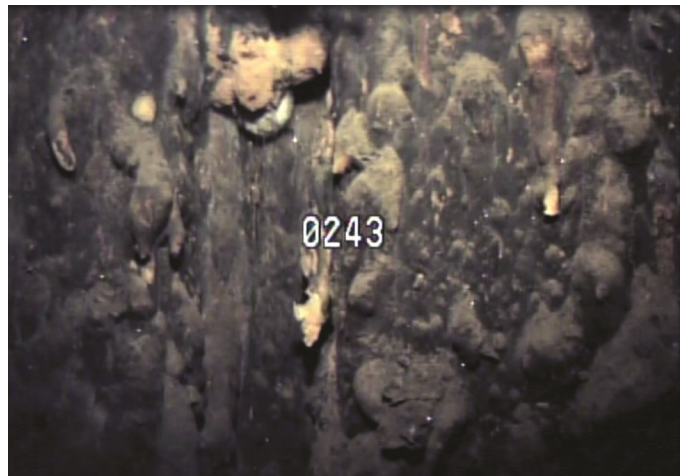
Well video image showing heavy biological and scale fouling, completely covering the screened section of the well.
