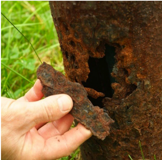
Hole in casing caused by corrosion.
