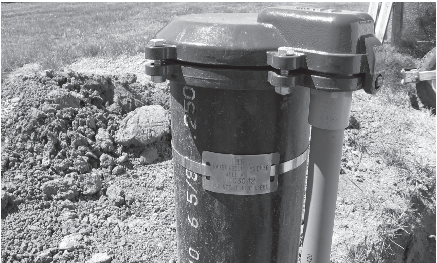
A metal well label, displaying the well ID number, should be on every well.
