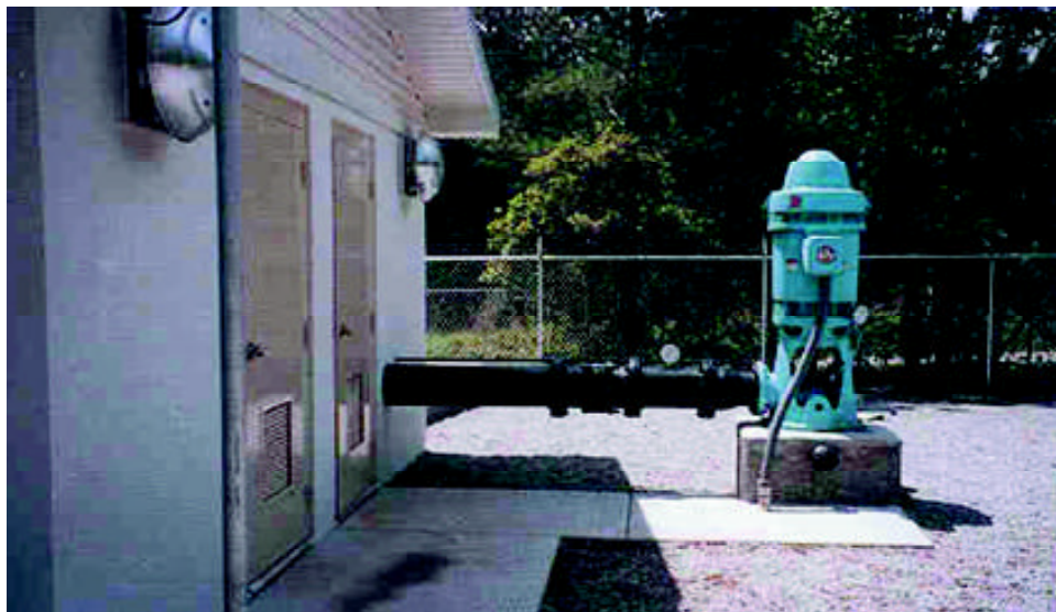
Water Supply Well in Butler County
