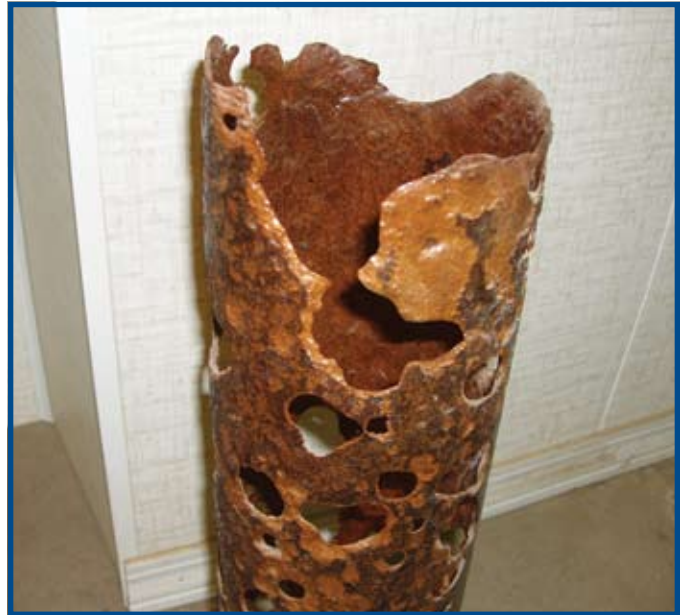
Figure 5. Corroded well casing.
