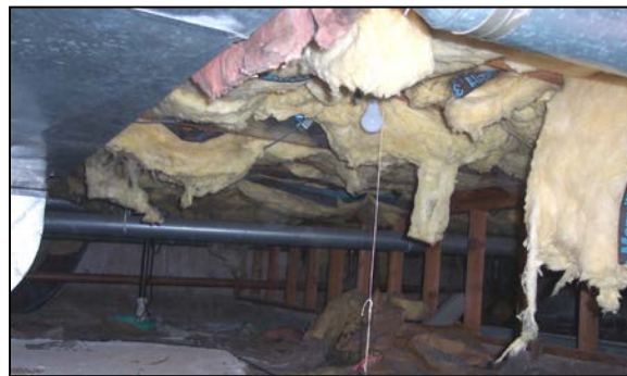
Figure 2. Vented crawl spaces often have poor insulation, no vapor control, and unsealed mechanical ductwork.
