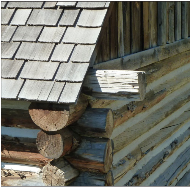
Figure 12. Support members extending beyond the roof overhang will eventually become wet enough to decay.
