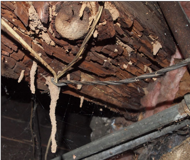
Figure 4. Support member with brown rot decay and termite mud tubes (Photo credit: Rachel Arango, USDA Forest Service, Forest Products Laboratory).
