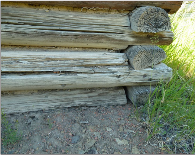
Figure 10. Placing logs directly on the ground ensures that decay will occur.
