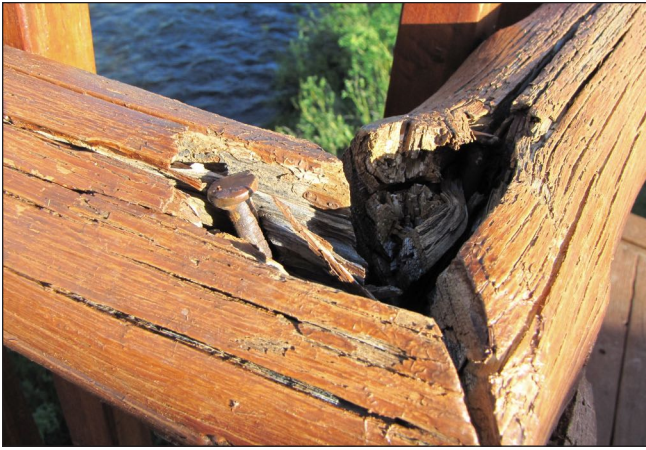
Figure 13. External components such as deck railings that are not protected by the roof overhang should be pressure-treated with a long-lasting wood preservative.
