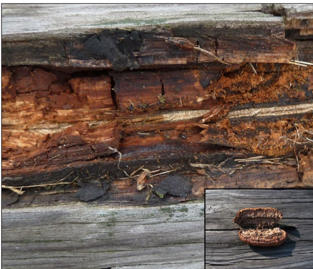
Figure 3. Brown rot fungi can cause serious structural damage to log homes if sufficient moisture is present in the wood. Often, the damage is concealed within the log and the first exterior sign of decay is a fungal fruiting body (inset photo).
