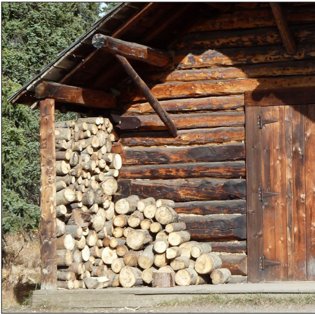
Figure 14. Firewood or other wood debris piled against cabin walls increases the likelihood of decay and insect attack.
