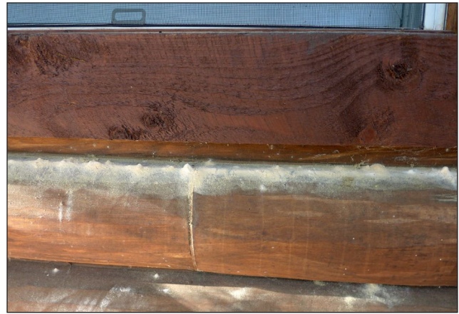
Figure 7. Powderpost beetle infestations produce fine, flour-like powder below small exit holes.
