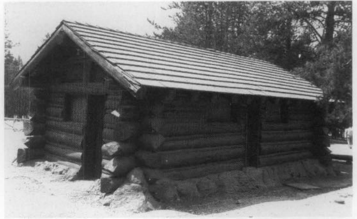
Fig. 18. Exposed roofing members of Rustic style buildings such as this structure at Yellowstone National Park are highly susceptible to deterioration. Photo: Laura Soulliere Harrison.
