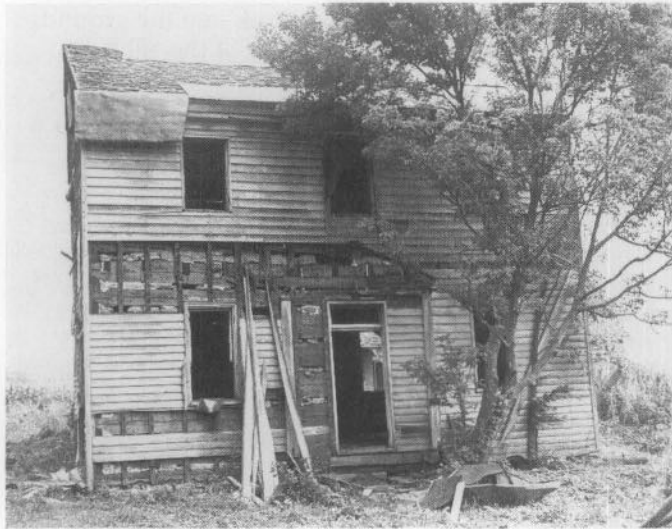
Fig. 14. Removal of the historic wood siding from the 1804 Zachariah Price DeWitt House in Butler County, Ohio, reveals that the clapboards were attached to vertical wood furring strips nailed to the logs. Photo: National Park Service Files.
