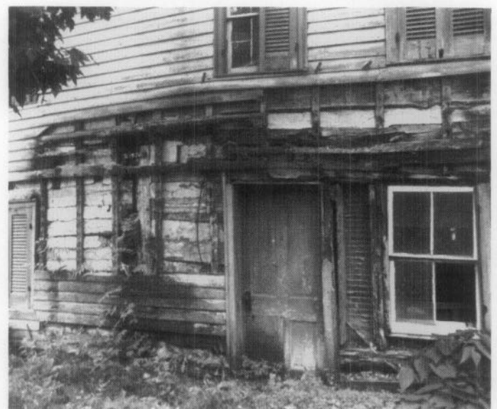
Fig. 17. Contact of this building's sill log with the ground has led to its decay, infestation by wood-destroying insects, and resulting building settlement. Photo: Anne Grimmer.
