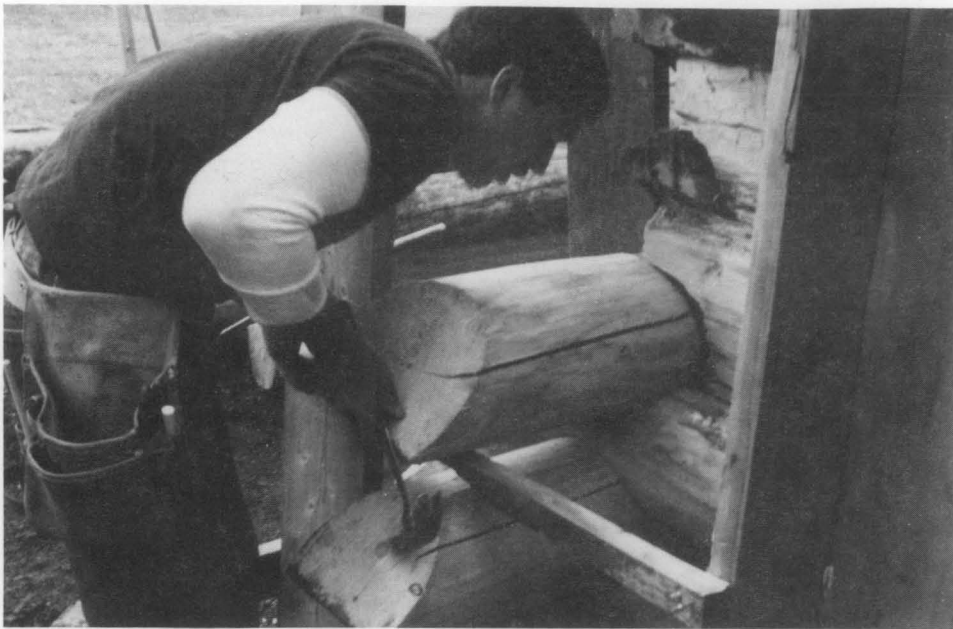
Figure 5. A framework or cribbing held the replacement crowns as they were fabricated. All the crowns had to be temporarily put in place to ensure a proper fit. Once stacked up, they were numbered to make sure they would be properly aligned at the time of anchorage. Photo: Harrison Goodall.
