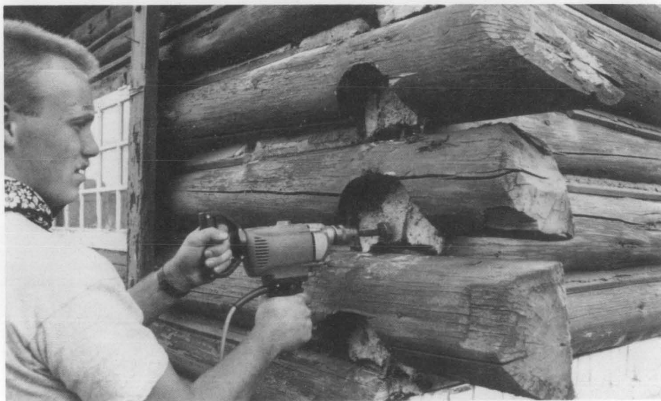
Figure 3. A plumber's bit was used to recess the crown back to the center line to create a flat surface for attaching the replacement crowns. Photo: Harrison Goodall.
