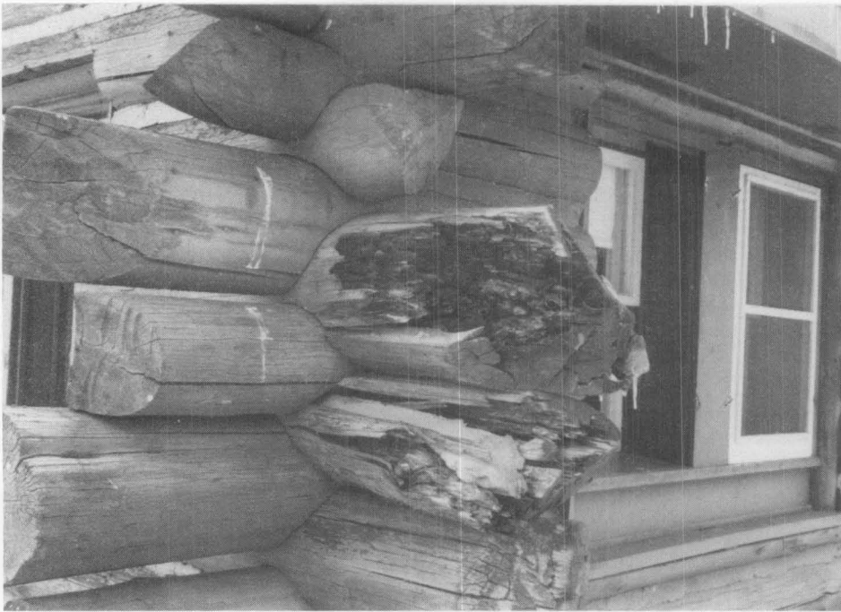
Figure 1. Typical deterioration of log crowns is seen at the Institute Building, adjacent to the Lamar Barn. This is the condition of many of the log crowns at the Lamar Barn prior to the repair and replacement work. Logs are notched at the corners. Photo: Harrison Goodall.
