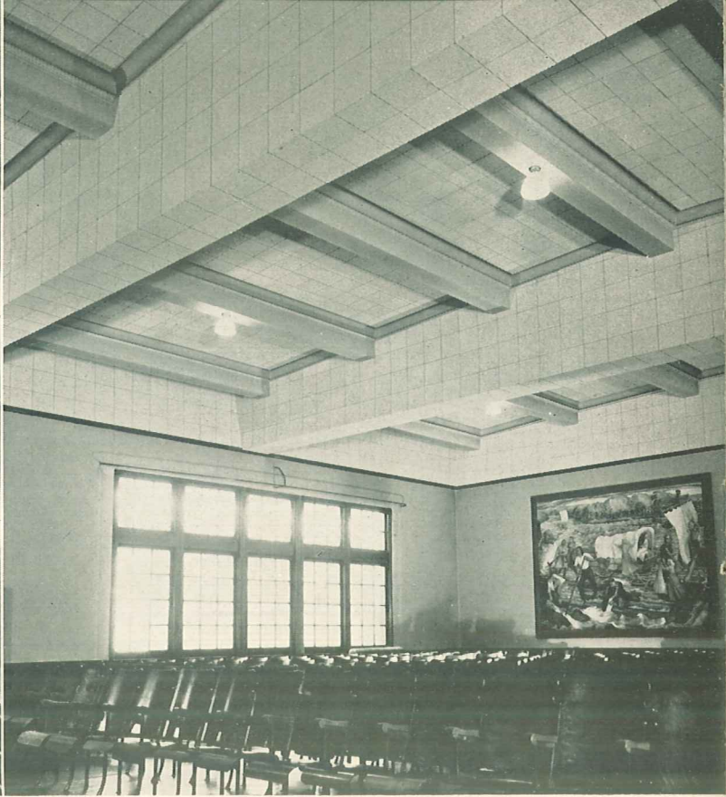
Fir-Tex acoustical treatment of this High School Auditorium is as effective as it is attractive.
