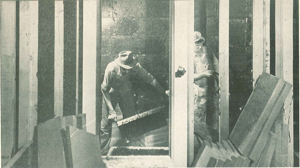
Above: The handy size Fir-Tex Refrigeration Block, held by two ice picks, has just been dipped in smoking hot asphalt and is slid into snug position.
