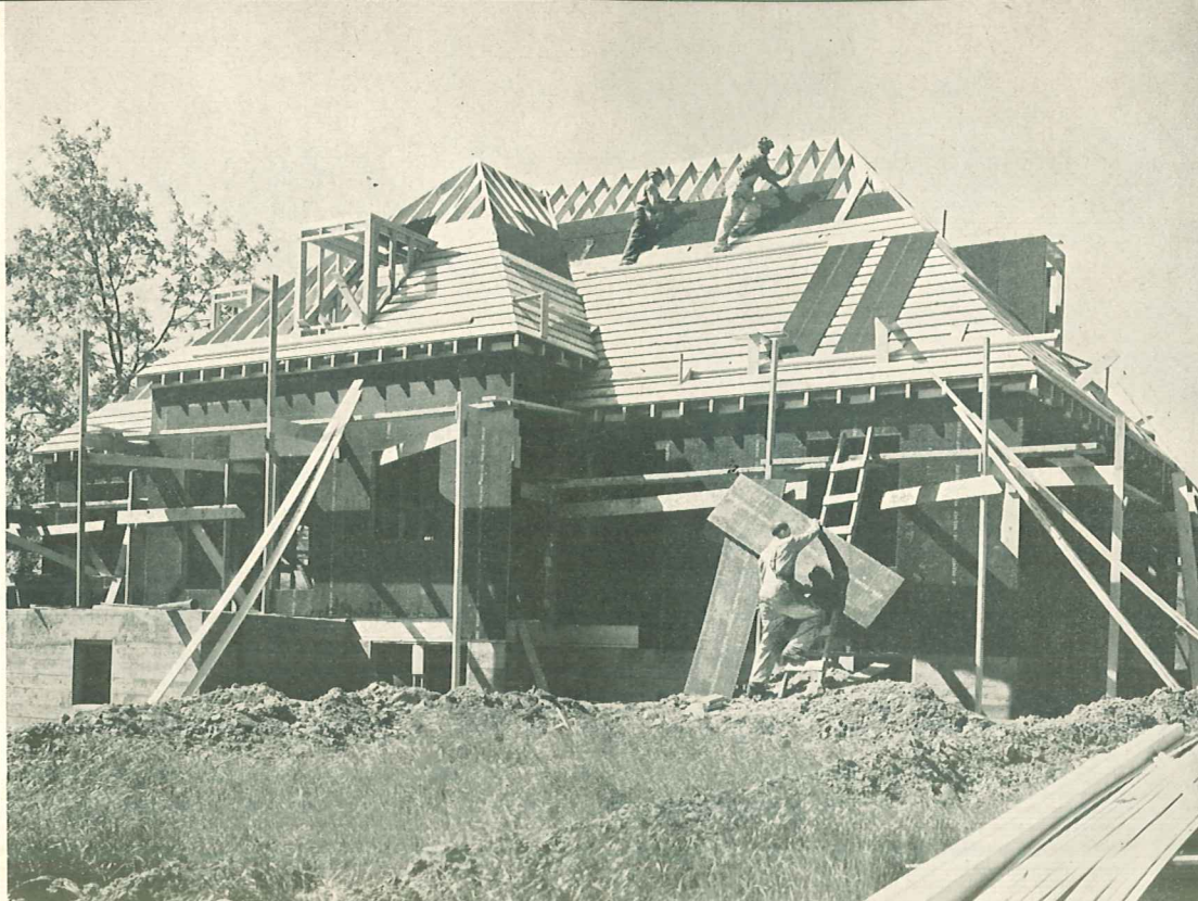
This picture illustrates the application of Firkote Sheathing on side walls and roof. This home will be entirely sealed from heat, cold, wind, dust and noise. It will be a comfortable home because it is adequately insulated.
