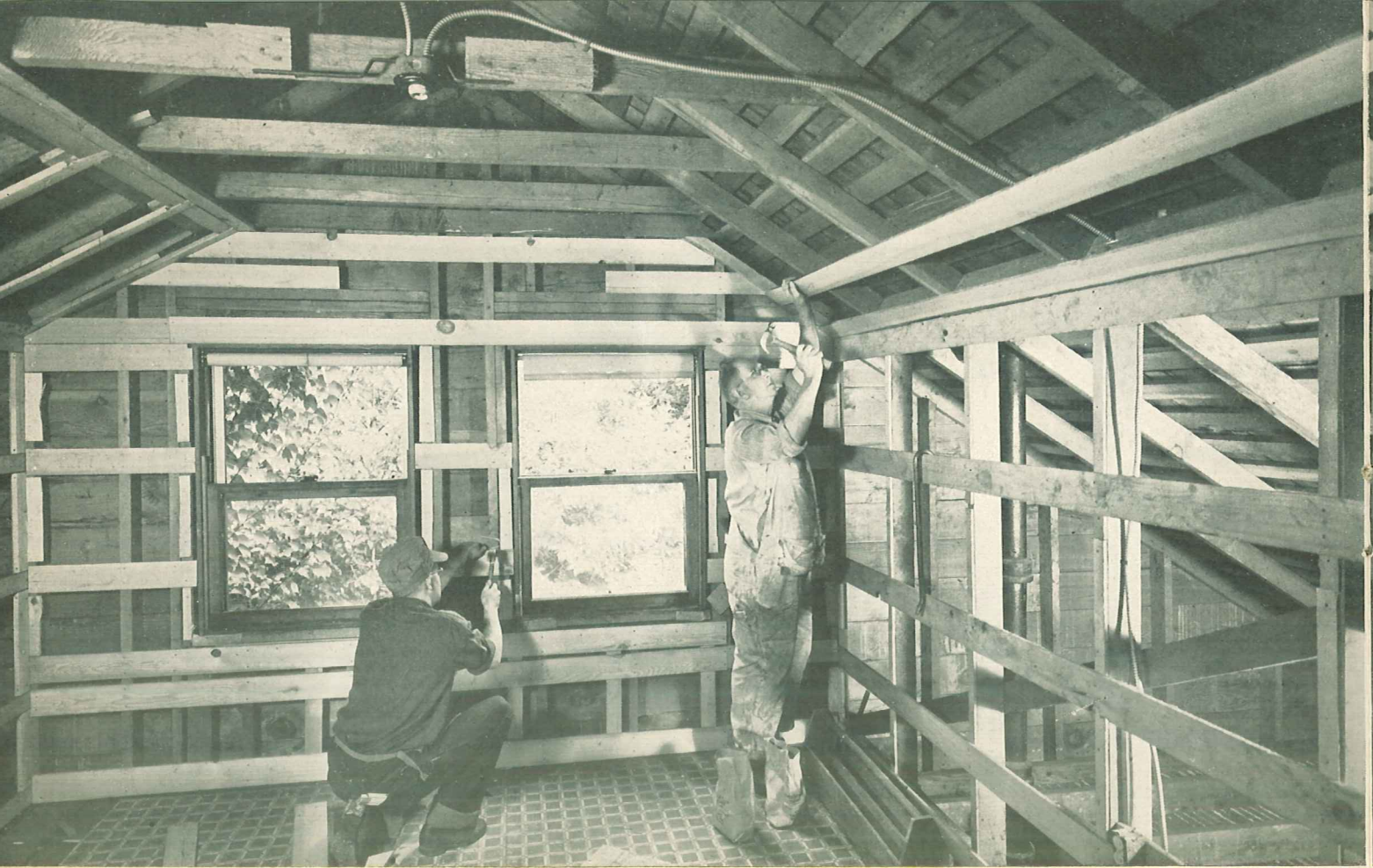
A Fir-Texed attic under construction. Note inexpensive lumber used as a nailing base.
