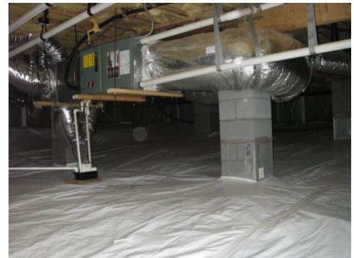
Raised HVAC System
