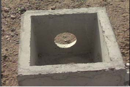
Figure 14. Typical distribution box.
