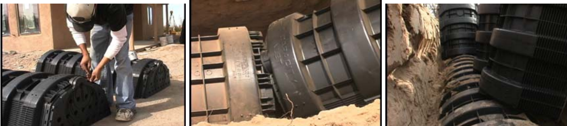
Figure 17. Screw in the end plate and then place the chambers in the trench in sequence.
