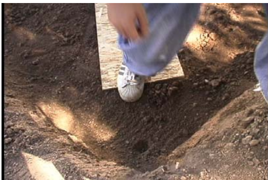
Figure 13. Trench bottom should be protected from extensive foot traffic using boards or planks.
