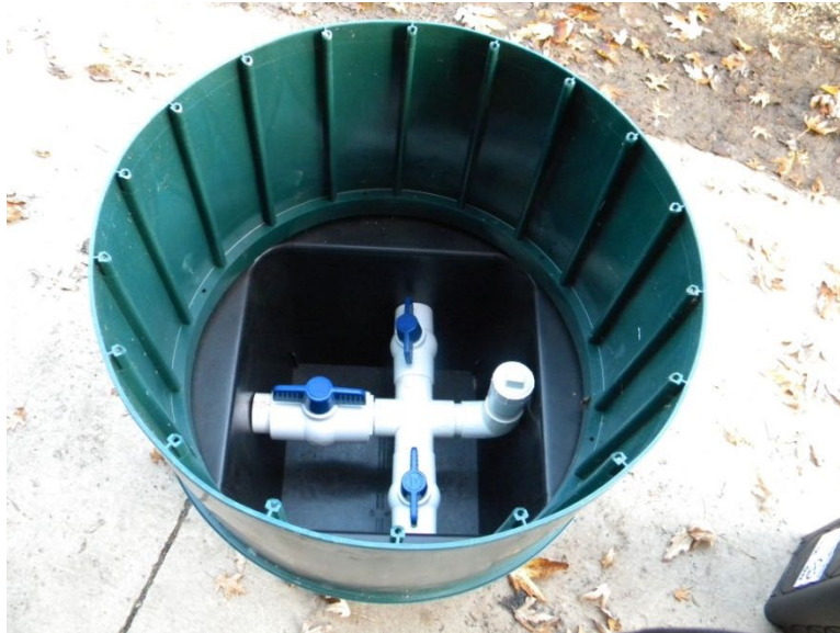
Figure 7. Service box within the manifold line
