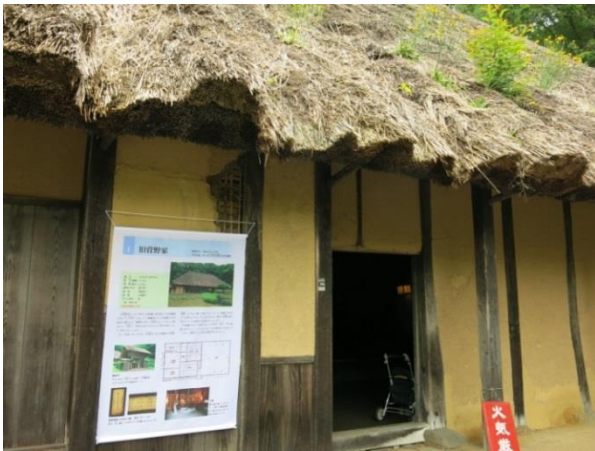
Fig 93. Roof on its process of decay.
