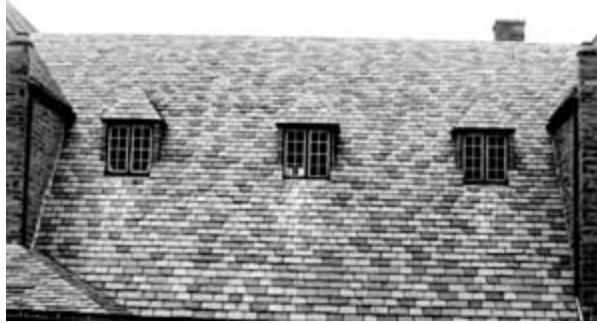
This graduated slate roof is composed of large, thick slates at the eave which are reduced in size and thickness as the slating progresses to the ridge. Photo: Jeffrey S. Levine.
