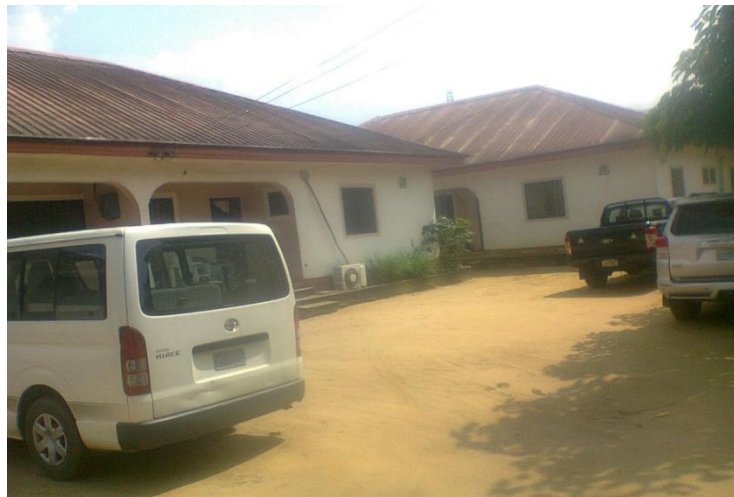
Fig. 5. Dark-Black Deposit on Colour Roofs in a Housing Estate in Uyo Town.
