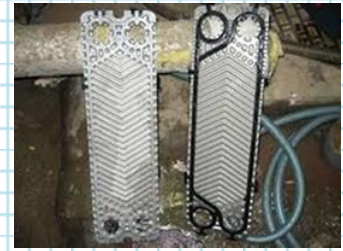
Plate heat exchanger
