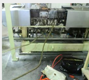
Ultra-fine cooling water piping
