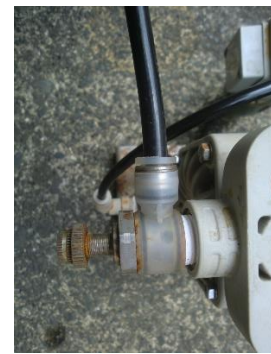
Pump outlet flow controller To set the flow as appropriate
