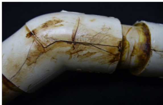
Image 1. Appearance of Incompatible Flame Retardant Damage
