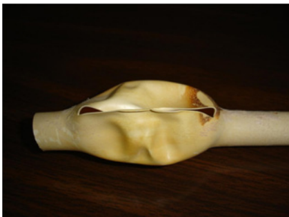
Image 24. Excessive temperature and pressure damage
