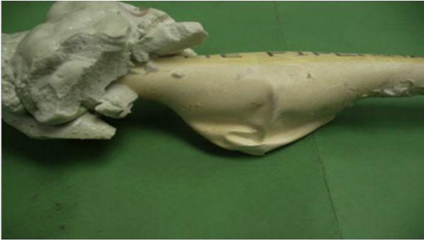
Image 3. Excessive heat damage caused by improper installation of two-part spray foam
