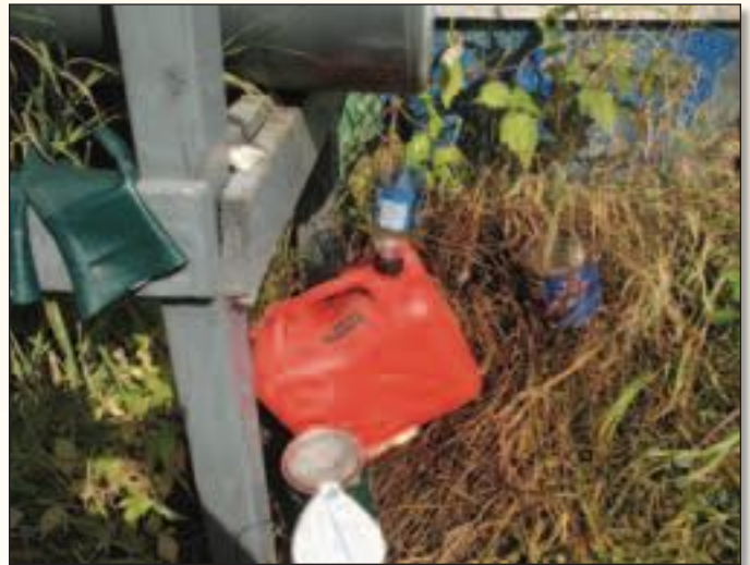
Attempt to capture oil leak. Note the dead vegetation around the tank.
