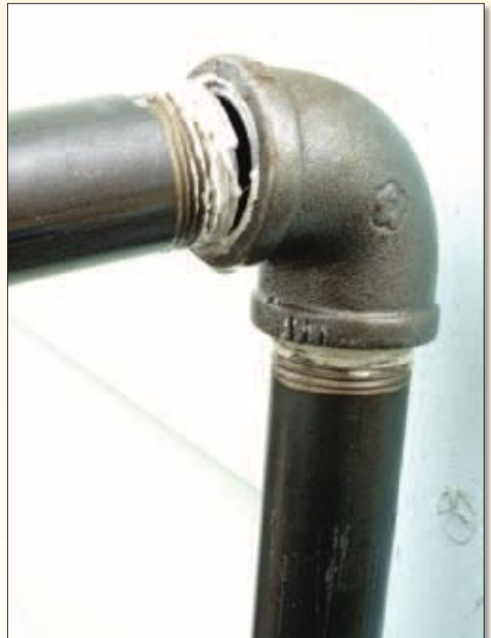
Broken fuel line at elbow due to stress from shifting oil tank.
