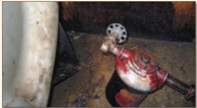
Broken valve on oil tank in basement.
