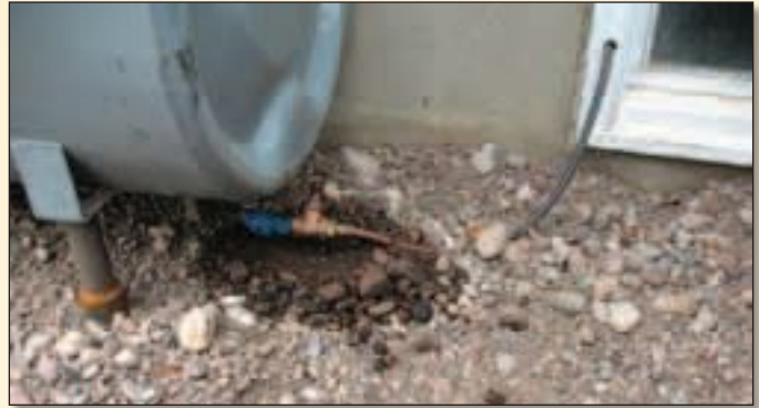
Small spill from a leaking valve.
