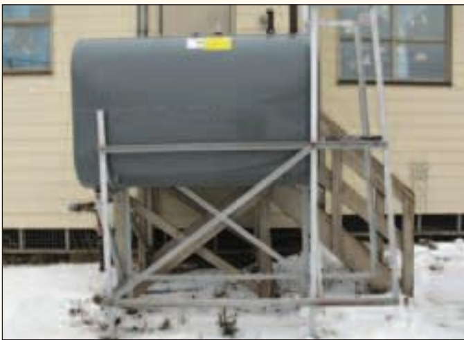
Epoxy-coated, 1,135 litre (250 gallon), single-wall steel heating oil tank on metal tank stand.
