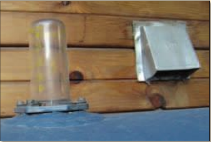
Oil level gauge. Note the empty tank.
