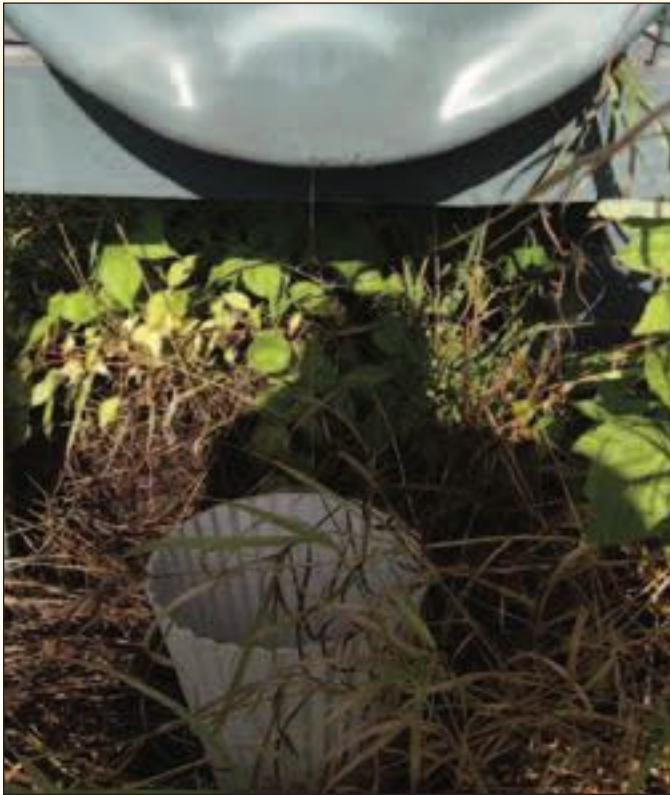
Leaking oil tank. Note the steady stream of oil from a pin-hole leak.
