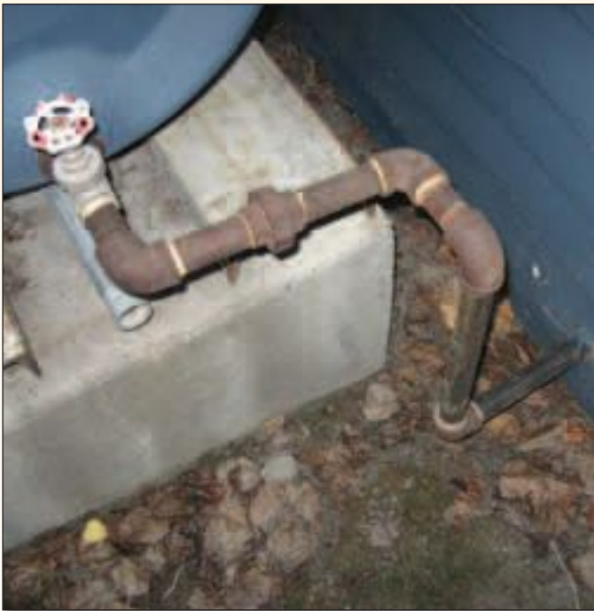
This type of fuel line is called a swing joint, which accounts for tank movement.
