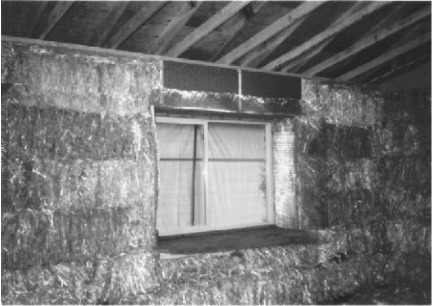
Figure 15.32 Window. ( Harvest Built Homes )
