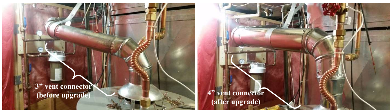
Figure 5.13. Three inch vent connector (left) upgraded to a 4 inch vent connector (right) in House CO1.
