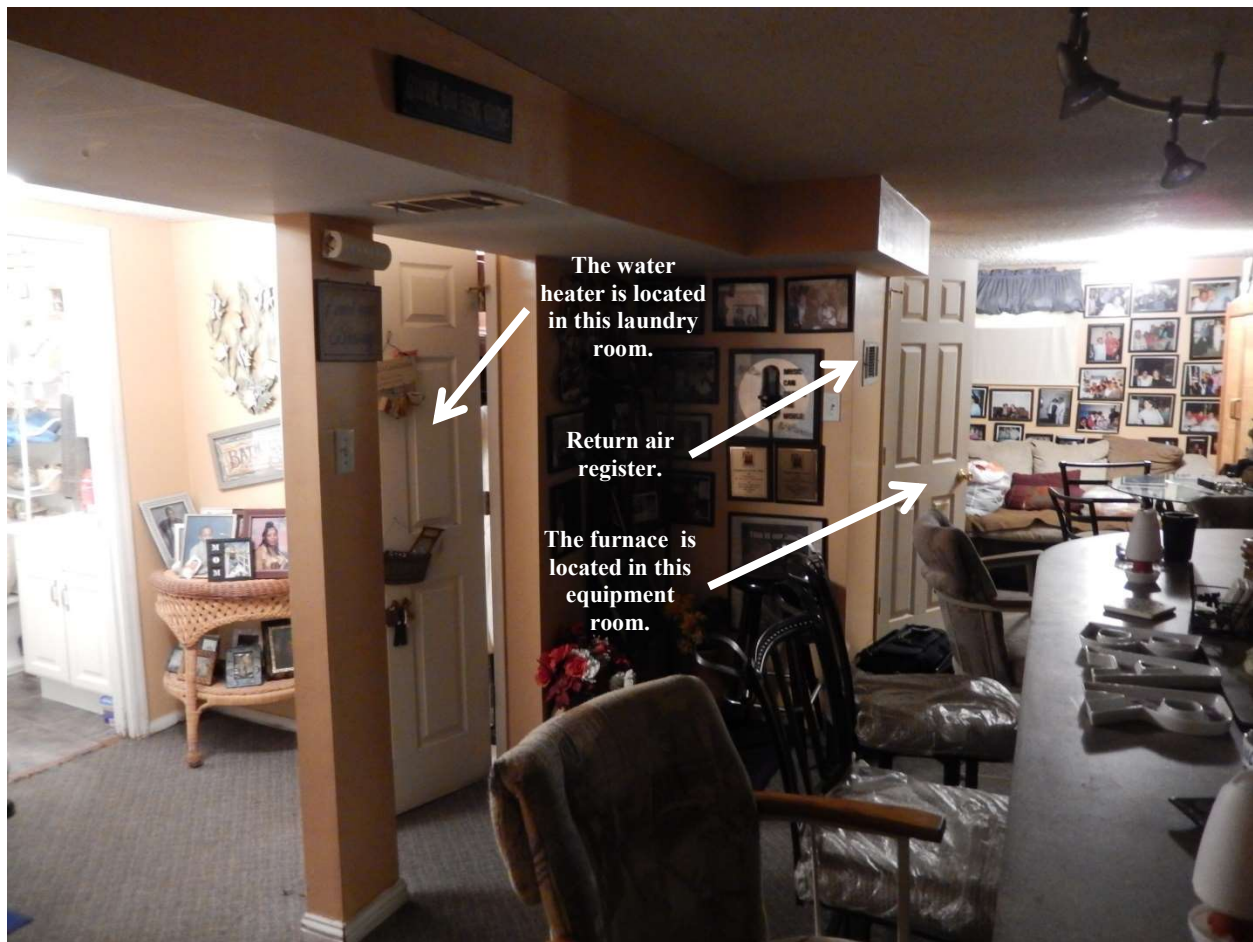
Figure 5.18. Basement equipment rooms in House MO3.
